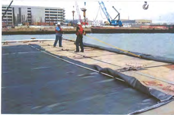
Deployment | The rolls of fabric were unfurled and floated into the bay from the deck of an 80-ft. x 60-ft. sectional barge. Photo courtesy of Triumph Geo-Synthetics.
