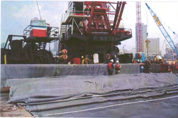
Rebar and prep/staging | The rebar was encased in PVC pipe capped at both ends. Photo courtesy of Triumph Geo-Synthetics.
