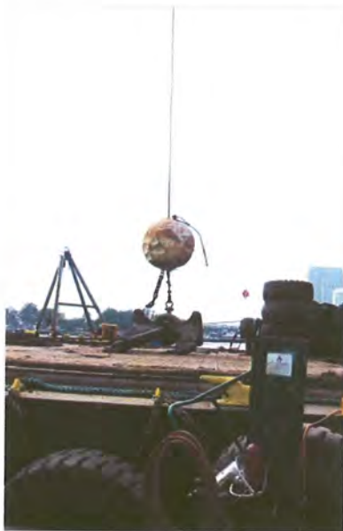
Crane with ball/anchor | When the derrick barge is moved, these 15-ft.-high anchors also have to be repositioned. Photo courtesy of Triumph Geo-Synthetics.
