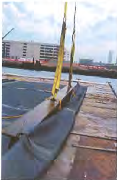
Prep and staging using an I-beam: To establish the start of a fabric run on the seafloor, the geotextile was attached to an I-beam. Photo courtesy of Triumph Geo-Synthetics.
