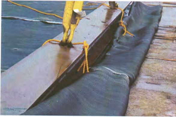
The positioning of the fabric was established with a global positioning system, monitored by the field superintendent and the crane operator. Photo courtesy of Triumph Geo-Synthetics.
