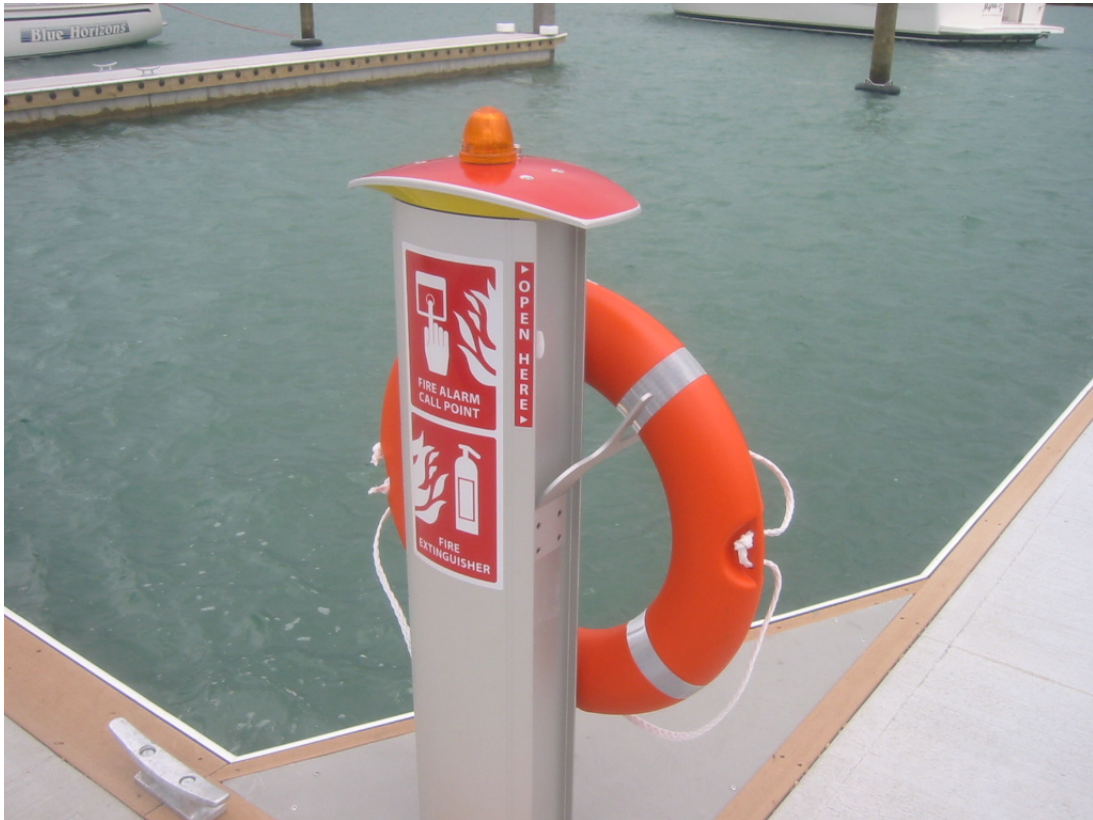
Photograph 3: Detailed view of buoyancy ring and fire point service bollard.
