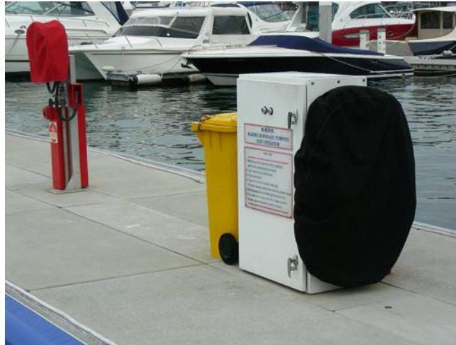
Photograph 7: Sewage Pump Out – View of Sewage Pump Out Point in Lockable Cabinet.
