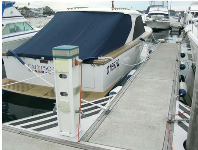
Photograph 5: Floating Structure – View along Finger Element of Floating Structure with Concrete Walking Surface with Service Bollard.
