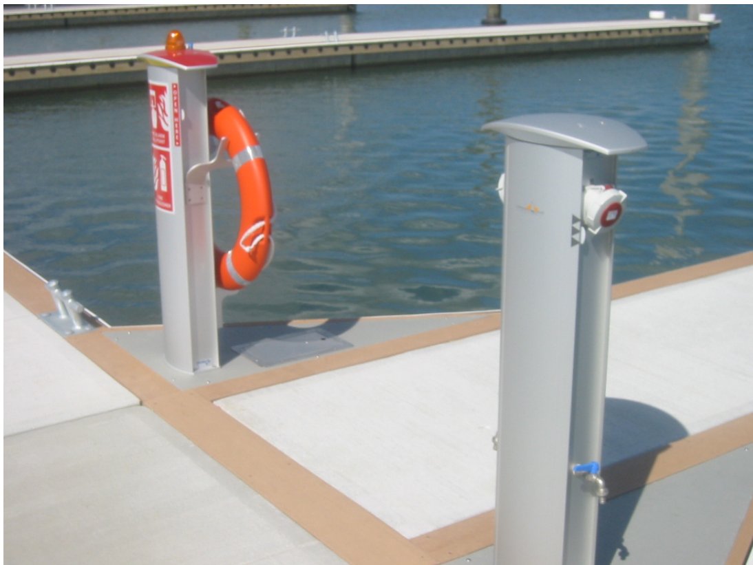
Photograph 2: Detailed view of services bollards.
