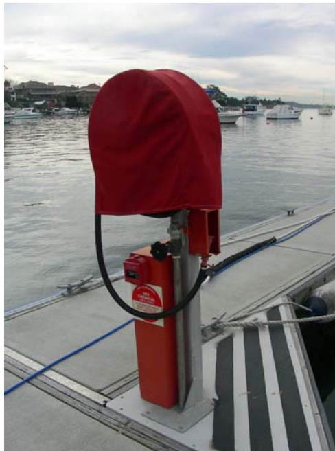
Photograph 6: Fire Services – View of Fire Hose Reel with Cover.
