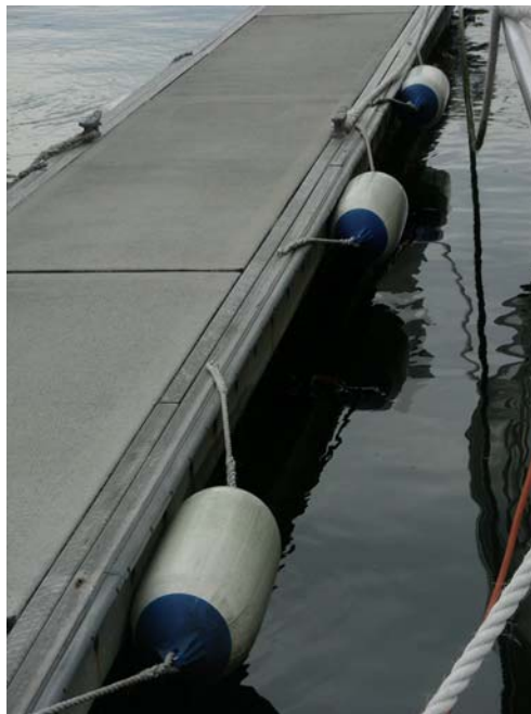
Photograph 10: Fenders – View of Pneumatic Type Fenders.
