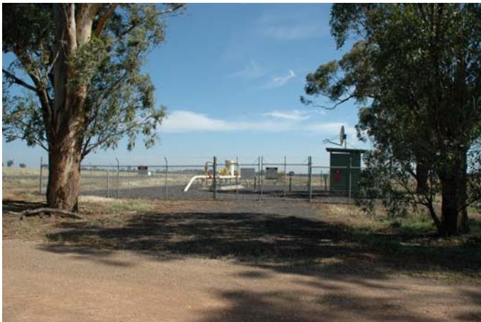
Figure 23: Alecstown offtake station
