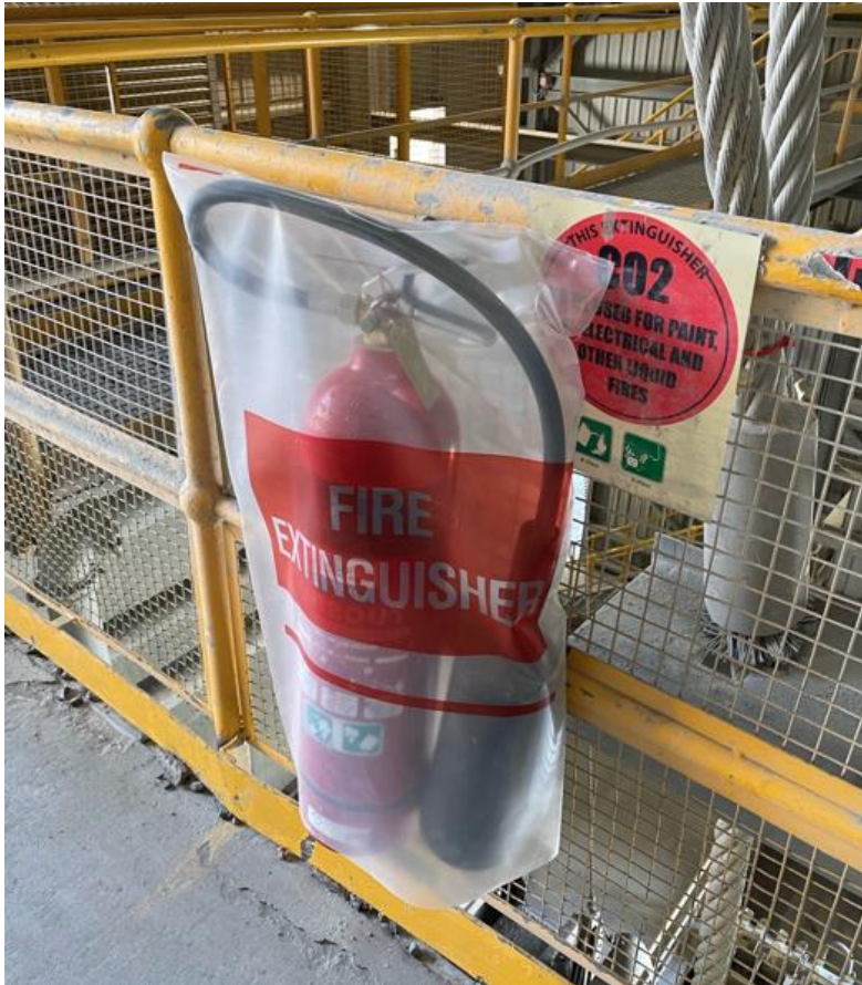
Plate 9 Tagged portable fire equipment available inside the ore processing facility
