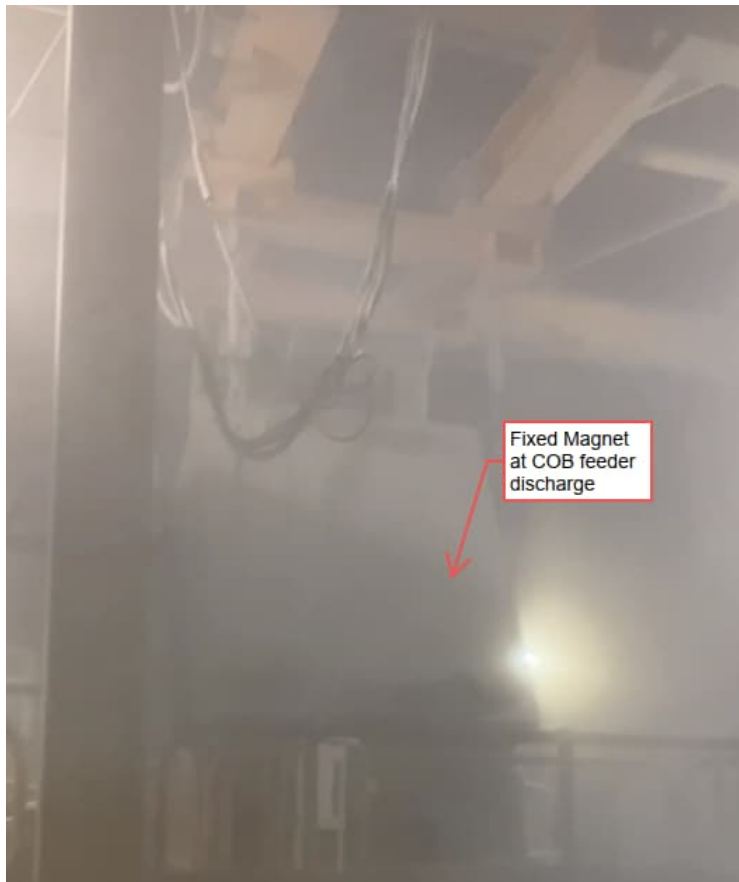
Figure 26 Typical Dust haze in the collection area
