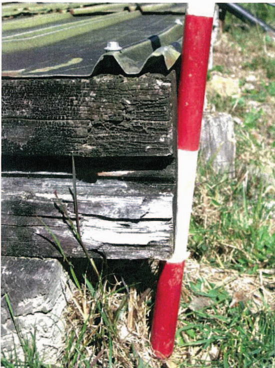
Detail of timber bearers with grooves on western side of platform (looking south).
