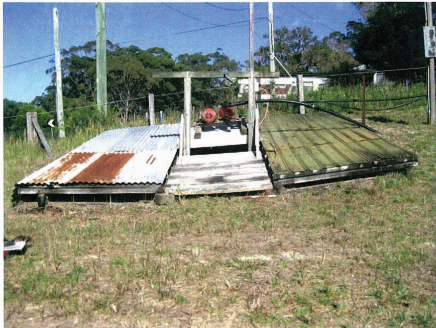
View of exterior of mine shaft (looking south) covered by timber, aluminium and iron sheeting supported by timber bearers. A water pump is located at the centre of the structure.
