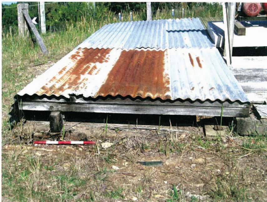
View of the exterior of mine shaft showing metal sheeting covering supported by timber bearers (looking south).
