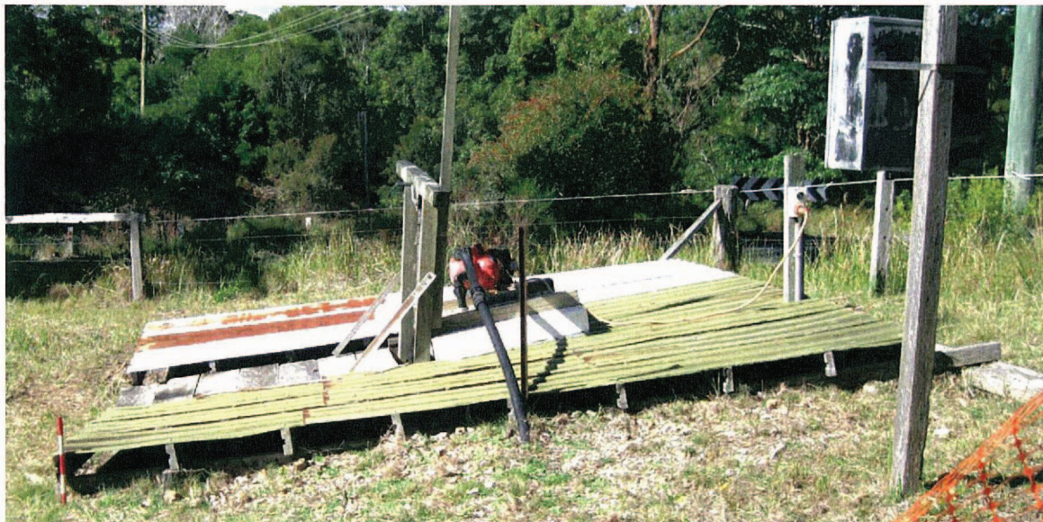
View of the exterior of the mine shaft (looking east) covered by timber, aluminium and iron sheeting supported by timber bearers. A water pump is located at the centre of the structure.
