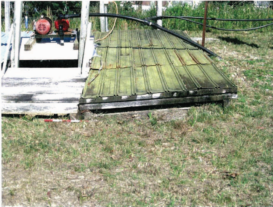
View of the exterior of the mine shaft showing metal sheeting supported by timber bearers (looking south).
