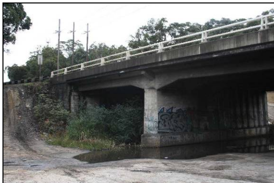
Plate 5: Kings Falls Bridge, upstream side. View of Appin approach, substructure and deck, facing north-west
