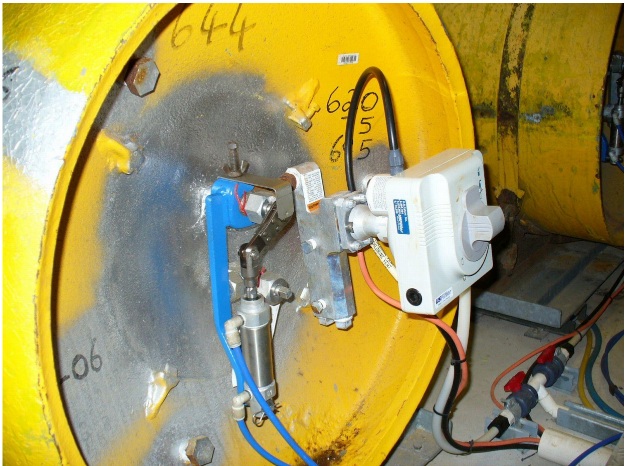
Chlorine drum connection detail showing Chlorguard unit and vacuum regulator. (Photo taken from Coffs Harbour City Council's Red Hill tank site chlorination plant)
