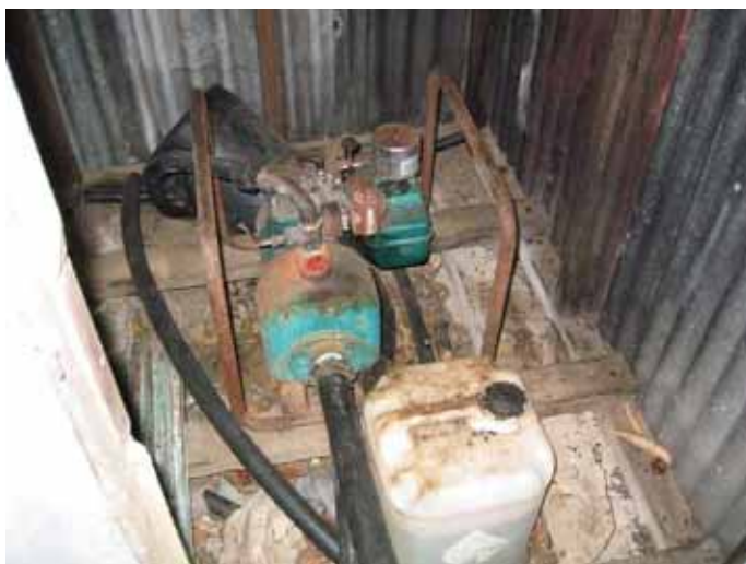
Photograph 9: Interior of small pump station adjacent to Orara River.
