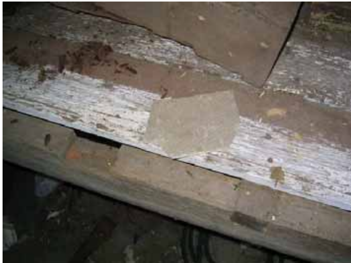
Photograph 4: Small piece of cement fibre sheeting potentially containing asbestos within garage / shed adjacent to large shed.
