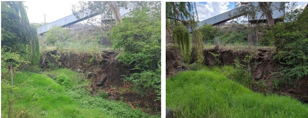
Plate 2. Erosion along Doughboy Hollow Creek
