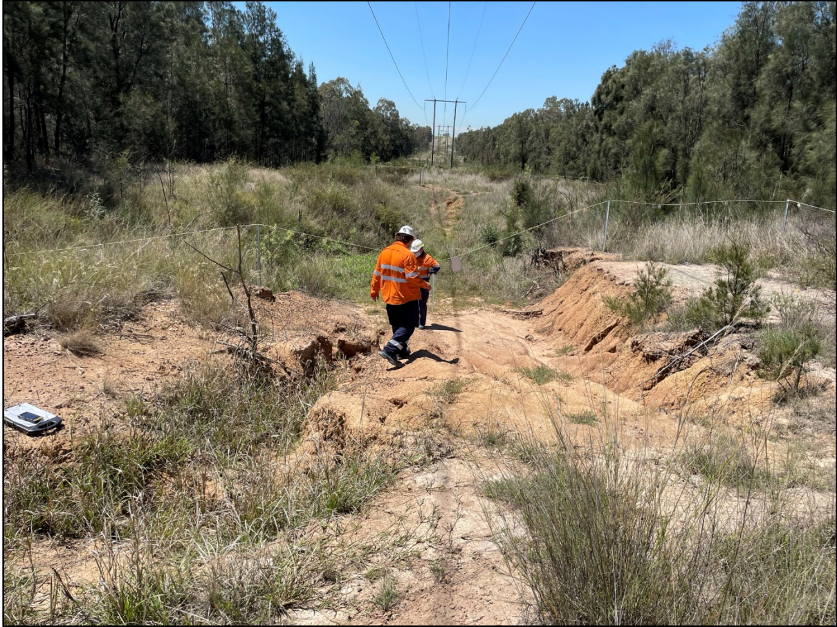
Example of erosion at site 37-2-0806
