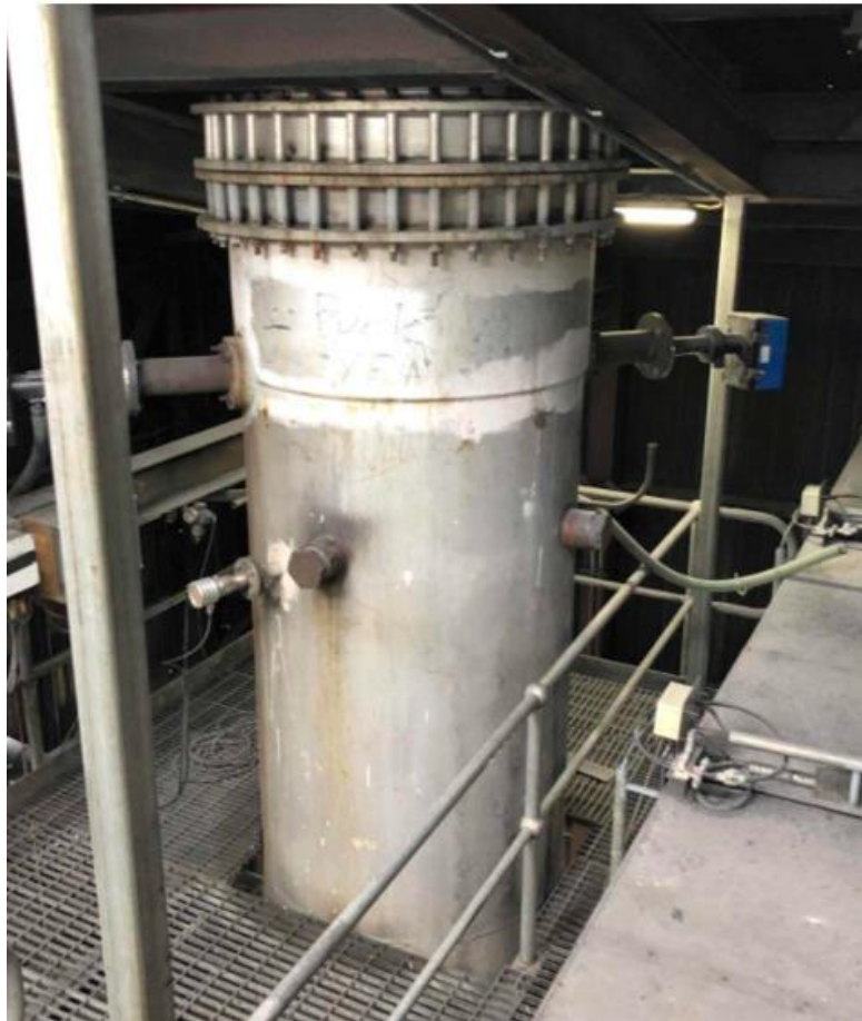
Figure 3. EPA ID 42 - Boiler 4
