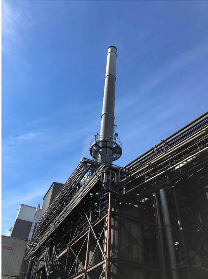
Image 1. EPA ID 35 - Boiler 6
