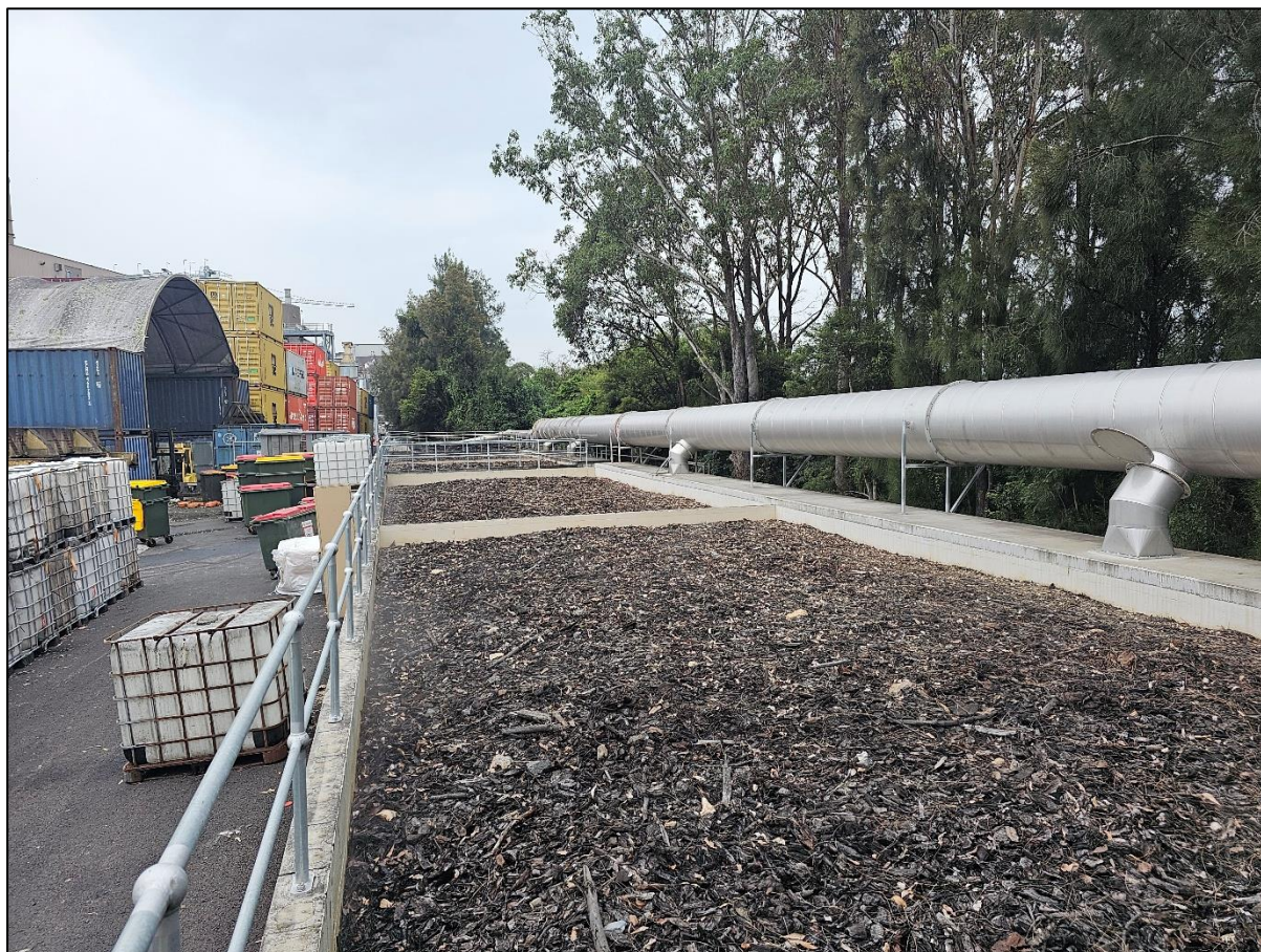
Photo 8.1 – A view of DDG Biofilters as found on 26 May 2025
