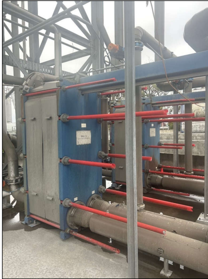
Figure 1 – Plant Heat Exchanger Photo – Source: Shoalhaven Starches
