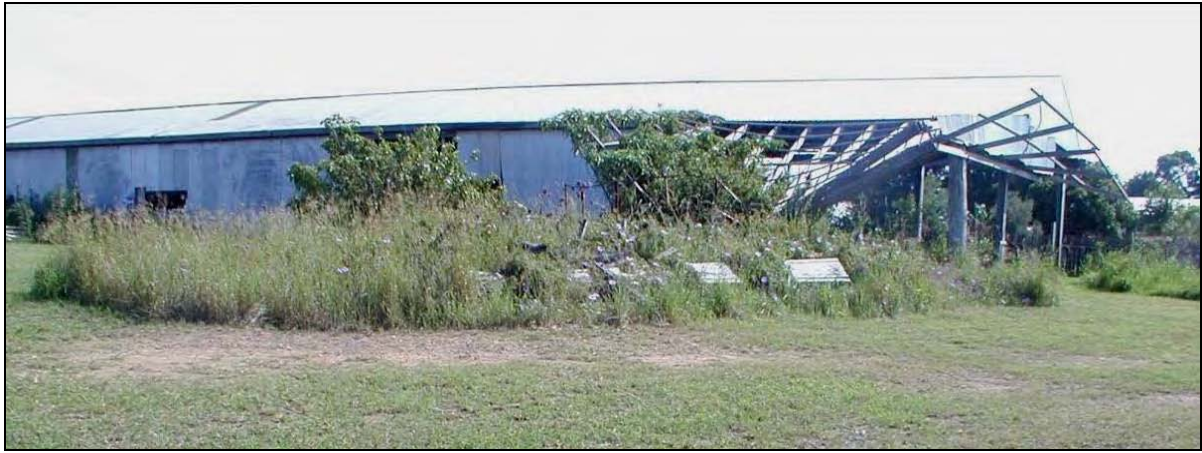
Plate 7.23 Former Jamieson's Timber Mill (KEH8). View of semi-collapsed building, looking northeast from the riverbank margin of the lot. This is the latest in a line of replacement sheds since the original mill was destroyed by fire in 1945.
