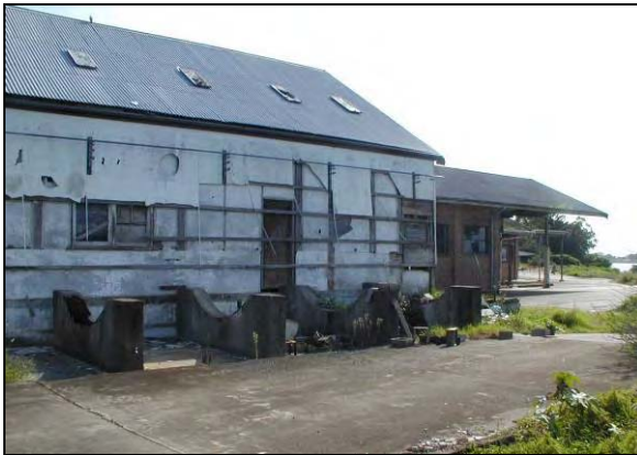
Plate 7.19 Side view of the derelict weatherboard Butter Factory building with the brick building to the rear – looking northeast
