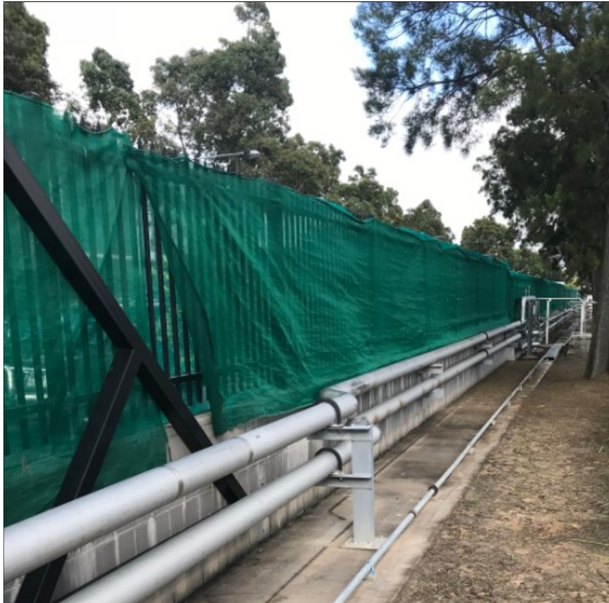
Existing GTP Infrastructure
