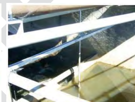
Photo 3a: Springvale drain at McPherson Street culvert V notch weir looking south.
