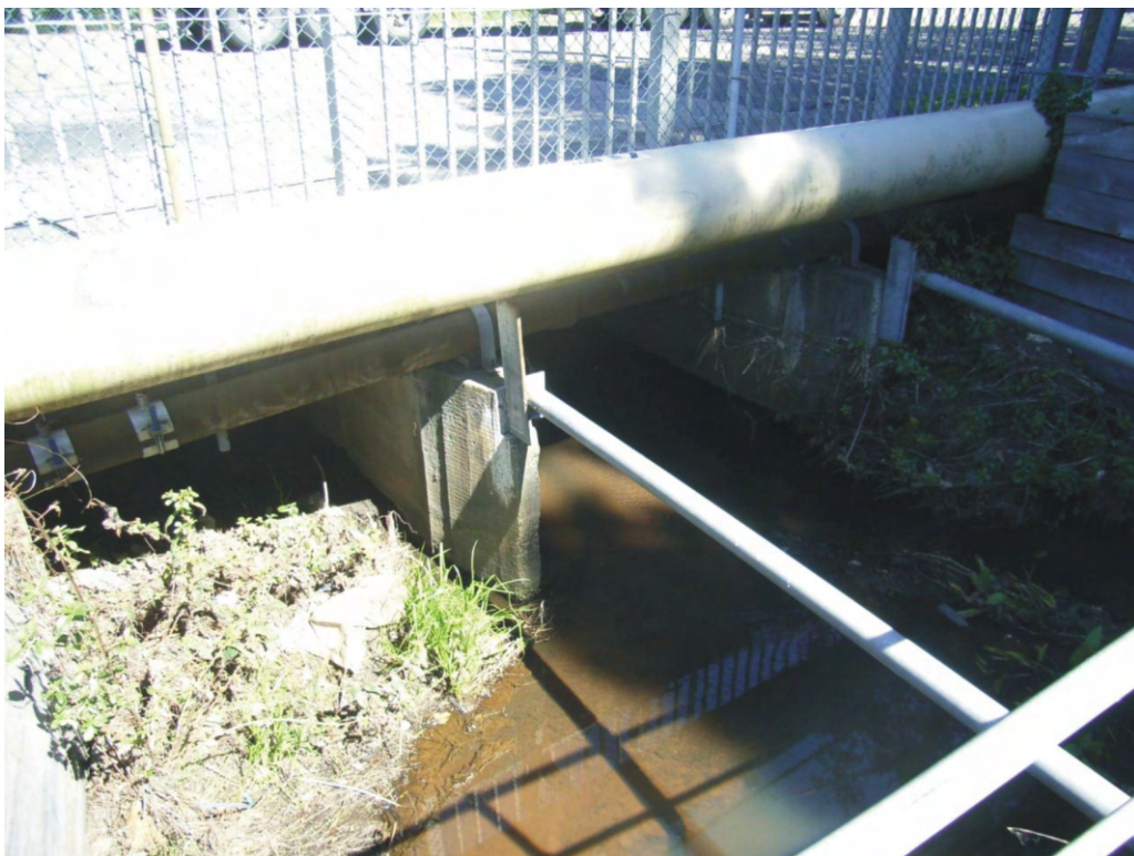
Photo 3a: Floodvaley drain at McPherson Street culvert looking south behind the trash rack.
