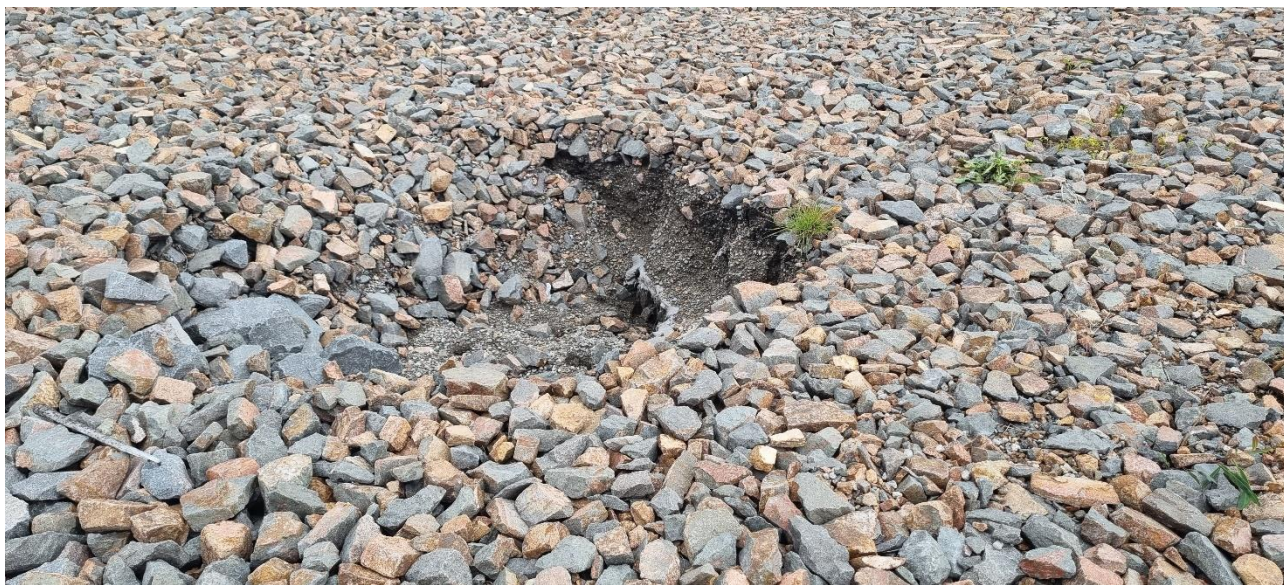
Photograph 5 - Sink Hole on Detention Basin D
