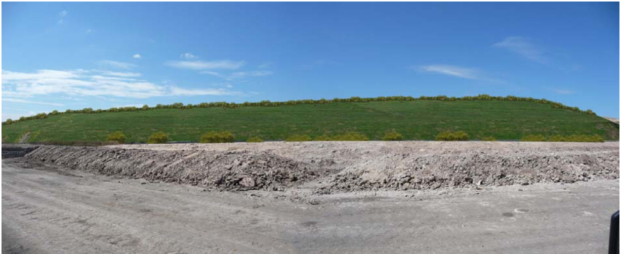
Photo 7B: Same view of the containment cell with height of cell raised by up to 4m (to RL 34), with landscape cover over cell and slopes
