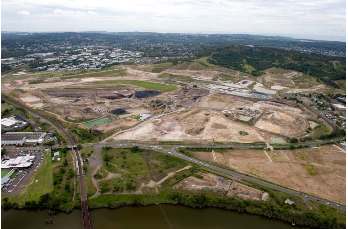
Figure.2: Aerial view from the east of the PCCS and IFL sites, Boolaroo (2012), with industrial buildings demolished and remediation of the site and Munibung Hill underway
