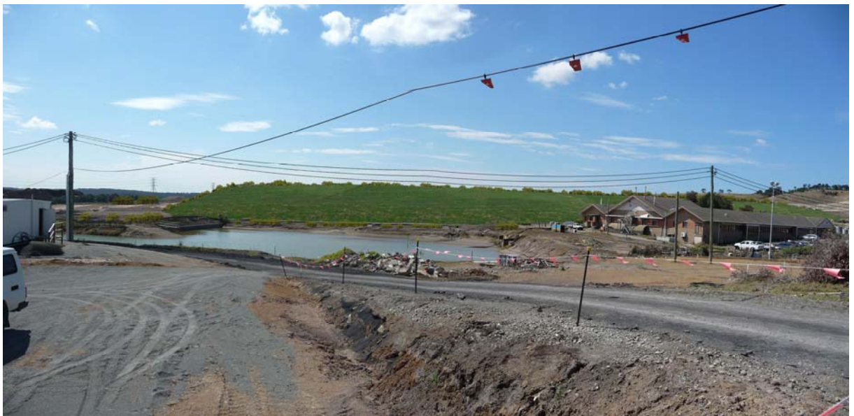
Photo 6B: Same view of the containment cell with height of cell raised by up to 4m (to RL 38), with landscape cover over cell and slopes
