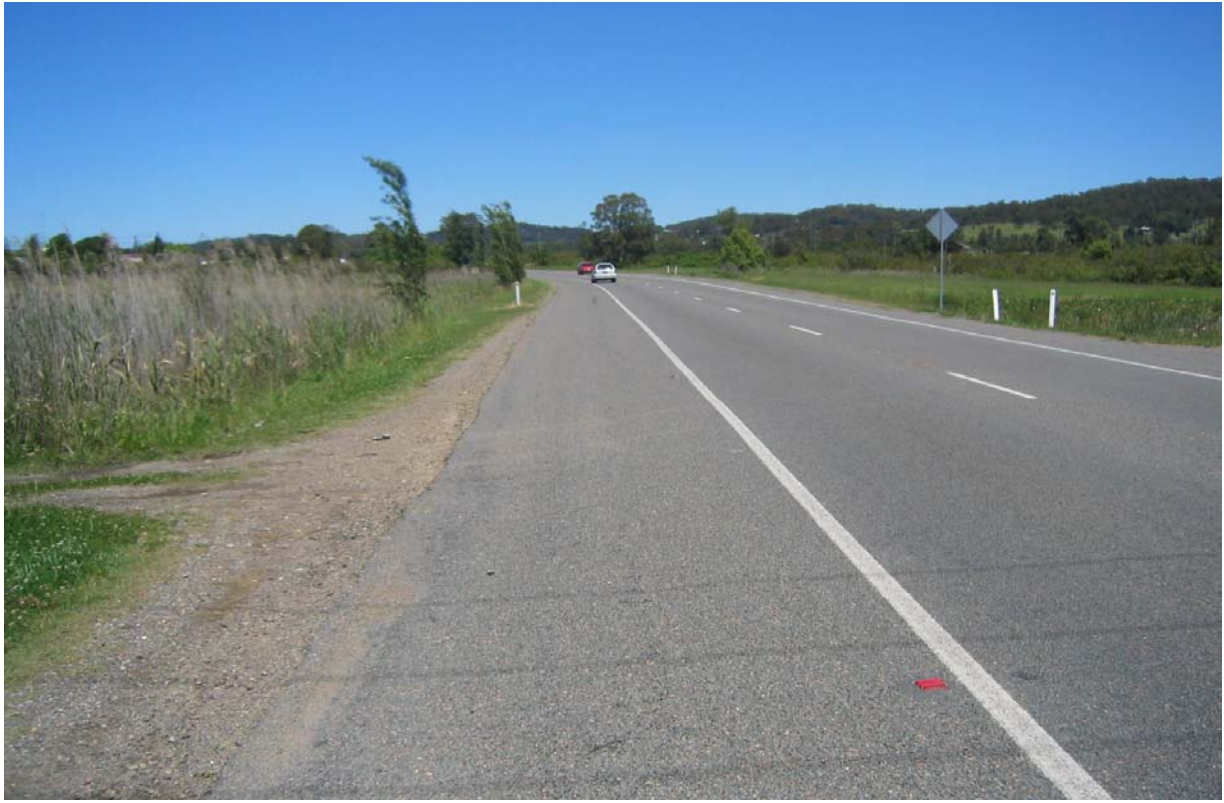
View looking south along TC Frith Avenue midway along the Triangular Paddock
