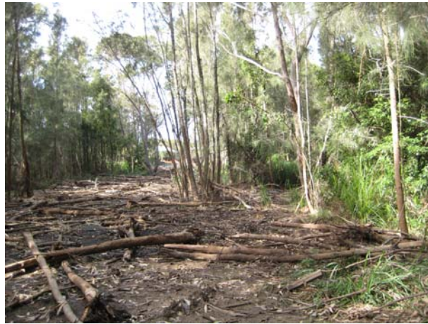
Photo 5: Clearing in proposed Lot 158 undertaken by Shoalhaven City for the sewer line
