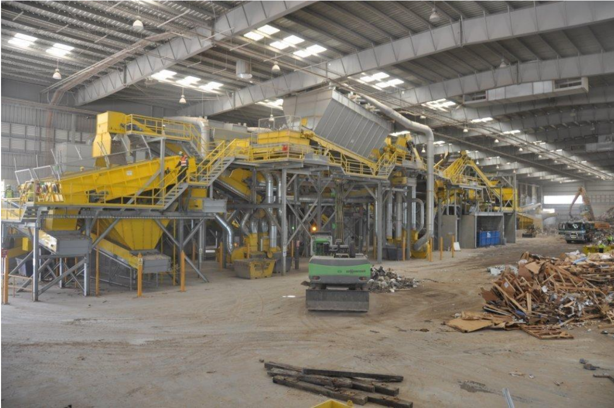
FIGURE 5 – VIEW OF PLANT INSIDE THE MPC (FROM THE SOUTHERN END) SHOWING THE CONVEYORS WHICH ARE ELECTRIC-DRIVEN
