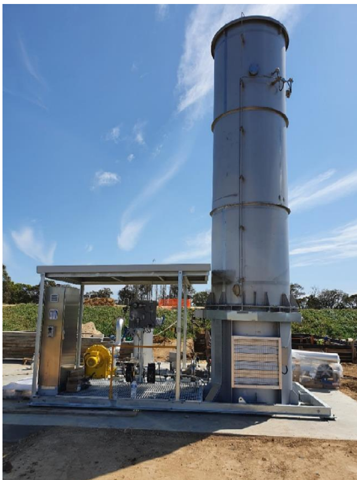
Figure 5-2: Example of the model OEF-300 flare installed in Western Australia.
