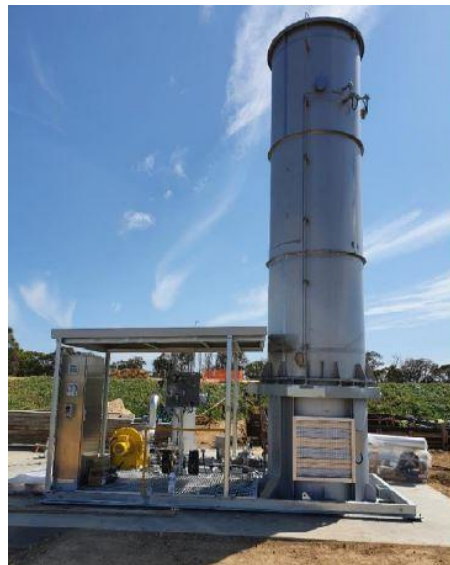
Figure 4 | Example of LFG flare
