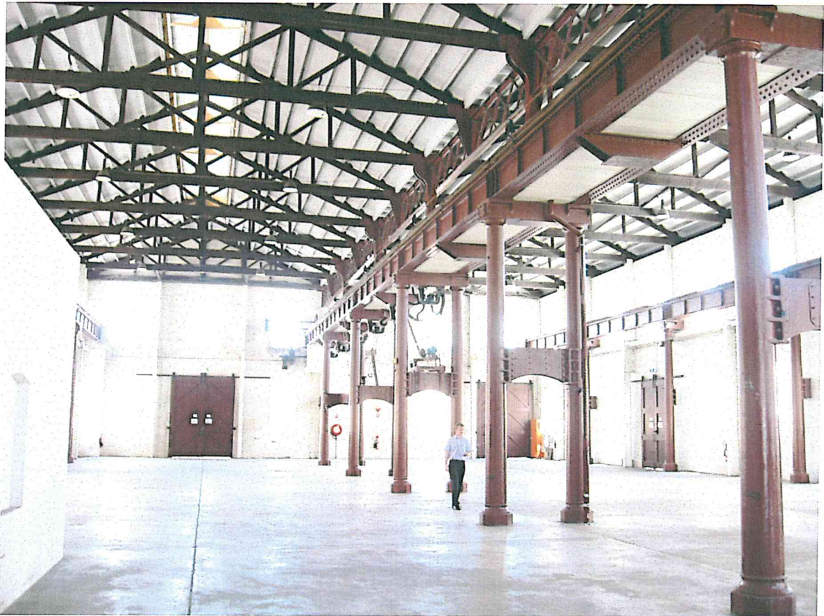
Figure 2 — Interior of the Boiler Shop in 2008, showing the cast iron columns that support the Craven crane.
