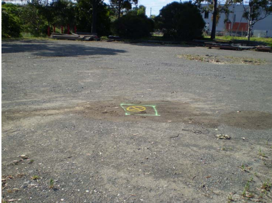
Photo 12- Localised staining noted in the unsealed gravel/roadbase area west of the warehouse (sample location TP1).
