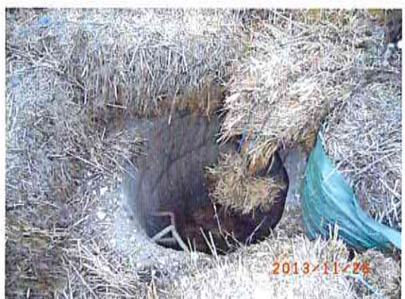
Photo # 163: Stormwater hole surrounded by hay bales as a sediment trap. No lid present.
