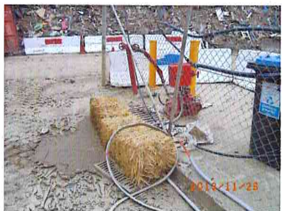
Photo # 178: Drainage from the wheel wash area and sediment control hay bales.
