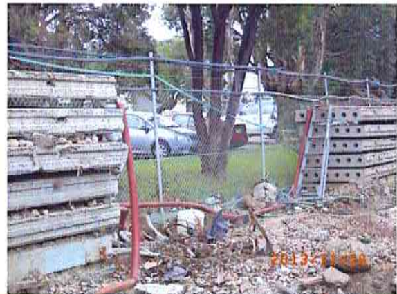
Photo # 267: Irrigation piping (black PVC piping at the top of the fence line) reportedly installed in the last two months to reduce dust emissions. Also note gaps in the temporary noise wall.
