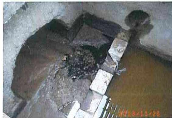
Photo # 100: Inside the final drainage point on site which flows to the Villawood culvert. Note sediment build-up, and black substance which may be oil.
