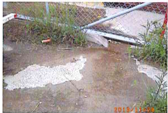
Photo # 132: Runoff from the waste processing area (Stockpile 1) running into the visitors car park.
