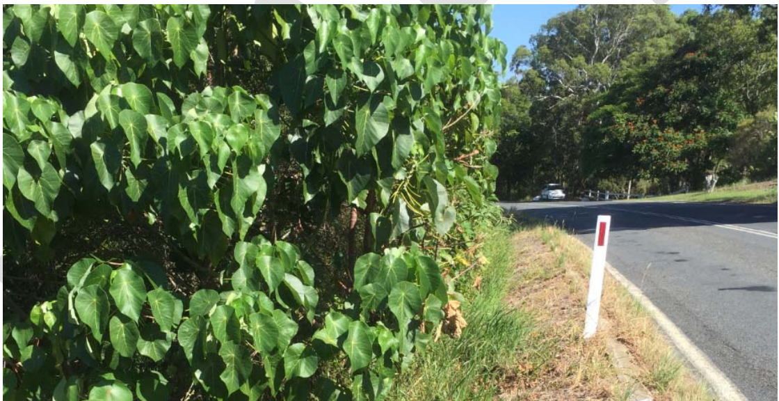
Figure 5: Example of existing 0.5m shoulder (with concrete kerb) next to a steep batter
