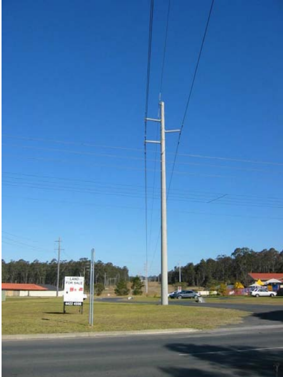
Figure 9.2 Typical 132 kilovolts transmission pole
