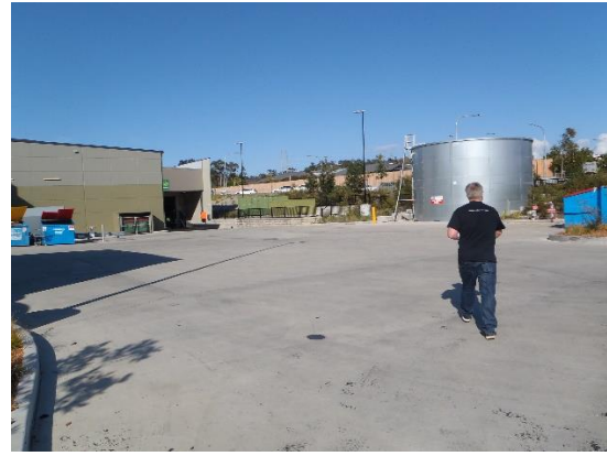
Photo 2: View of existing sprinkler water tank and substations from loading dock area Road – refer to Zone D in architectural drawings at Appendix A. Please note the change to include these existing features in Stage 1A.
