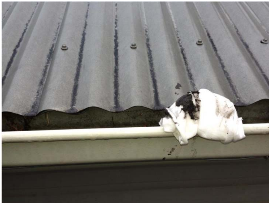
Black dust at 20 Yarraman Rd in roof corrugation valleys. The rag was lightly wiped in the guttering. This is the collection path for our drinking and house water
