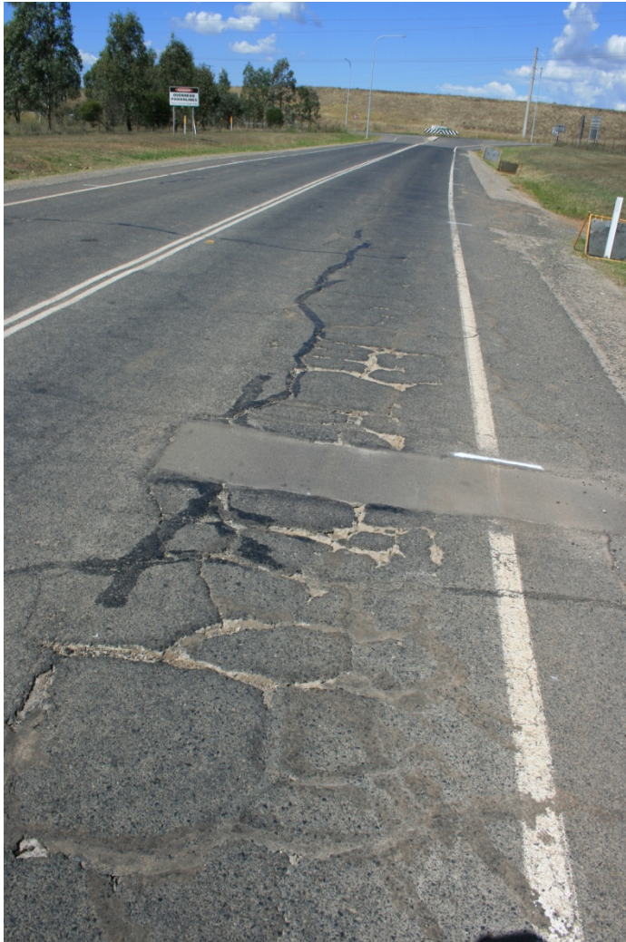
Figure 2.38 Poor pavement condition - Bengalla Link Road, looking eastbound toward its intersection with Denman Road
