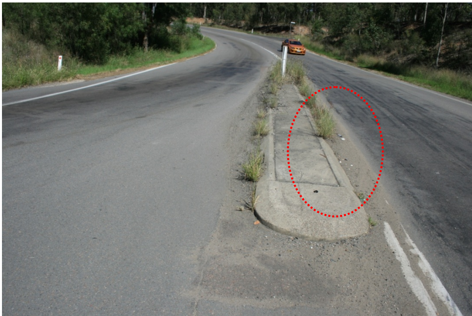
Figure 2.36 KEEP LEFT sign missing - Thomas Mitchell Drive, looking westbound from its intersection with the New England Highway
