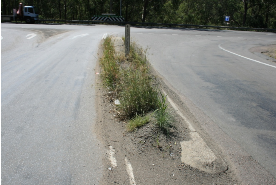
Figure 2.35 Median island overgrown by vegetation and partly covered by soil and gravel - Thomas Mitchell Drive, on approach to the intersection with the New England Highway
