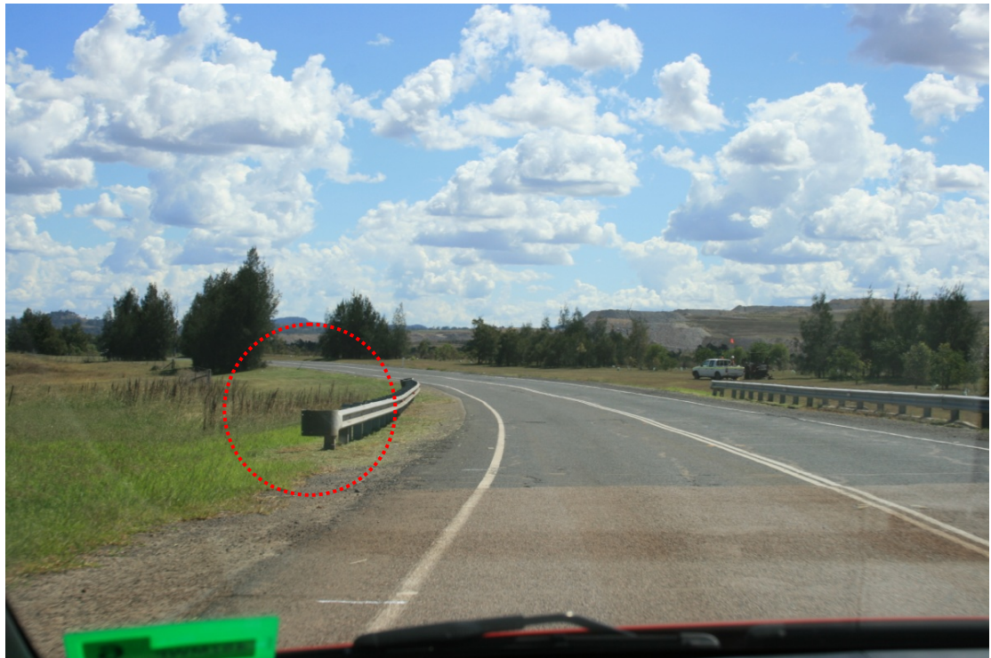
Figure 2.39 Unidirectional Hazard Marker is missing on the safety barrier – Bengalla Link Road, looking westbound
