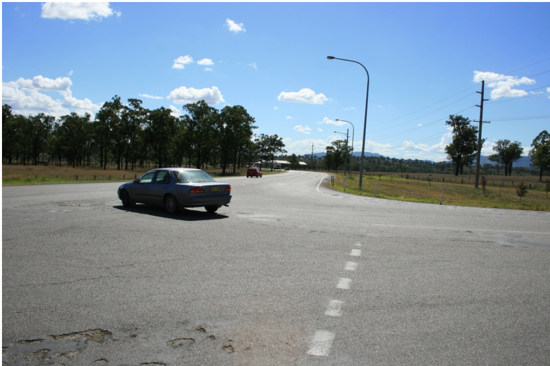
Figure 2.26 Potholes -Thomas Mitchell Drive/Denman Road intersection
