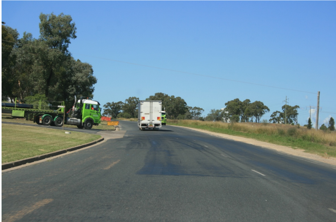
Figure 2.27 No edge line painted - Thomas Mitchell Drive, looking eastbound
