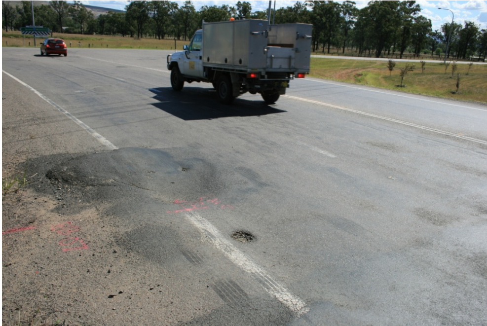
Figure 2.25 Potholes, uneven road surface and other pavement deficiencies - Thomas Mitchell Drive, looking toward its intersection with Denman Road
