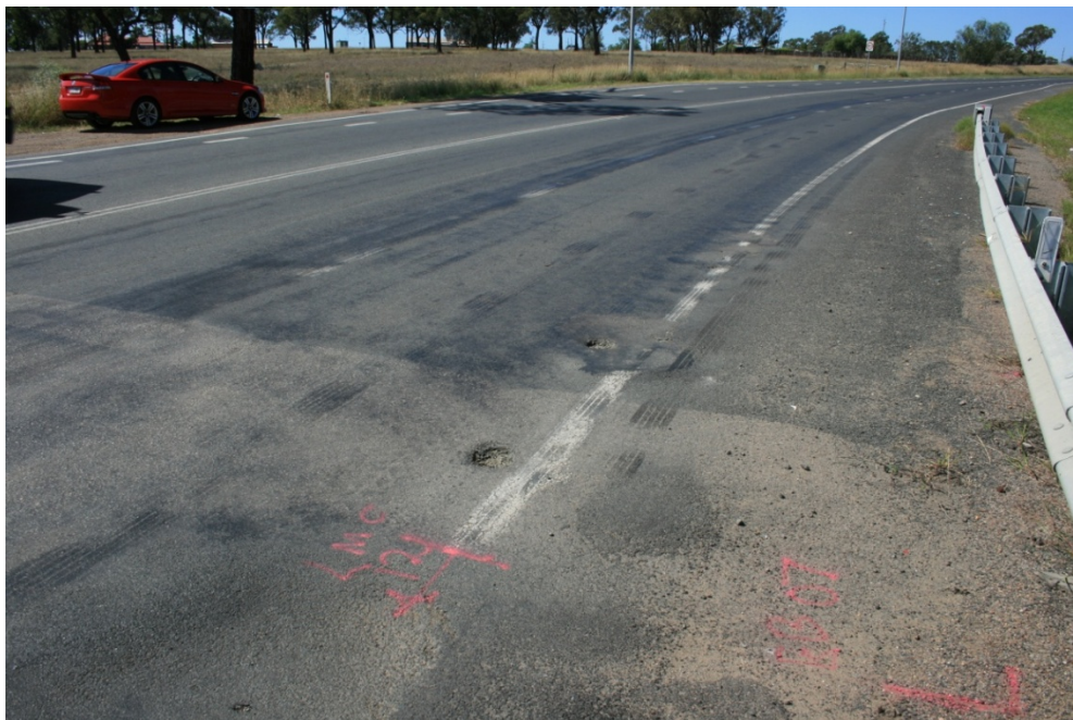
Figure 2.24 Potholes, uneven road surface and other pavement deficiencies - Thomas Mitchell Drive, looking eastbound from its intersection with Denman Road
