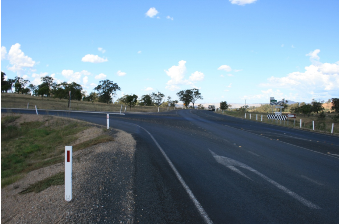
Figure 2.23 No sufficient contrast between the road markings and the pavement - Wybong Road/Bengalla Link Road intersection
