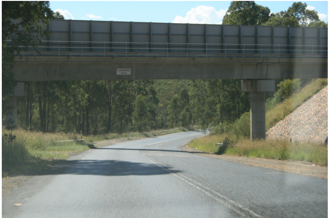
Figure 2.31 Substandard curve with no sufficient delineation provided - Thomas Mitchell Drive, looking eastbound
