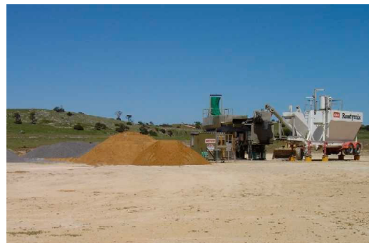
Plate 3.3 Typical Portable Concrete Batch Plant
