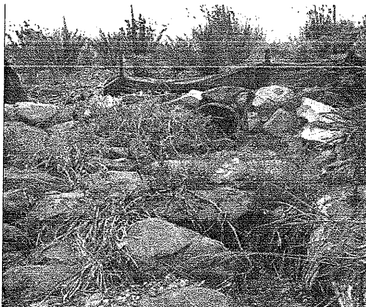
Figure 2. Rip-rap outlet structure with vegetation growing in voids between rocks.
