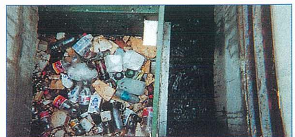
Typical gross pollutants captured and retained in the Ecosol RSF 4000 Solid Pollutant Filter
