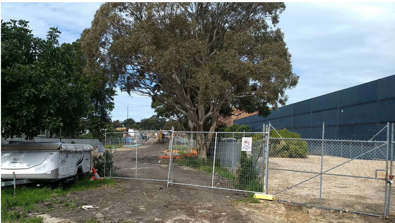
Figure 3 View of southern section of container noise wall following demolition of the B7 reel store - May 2020
