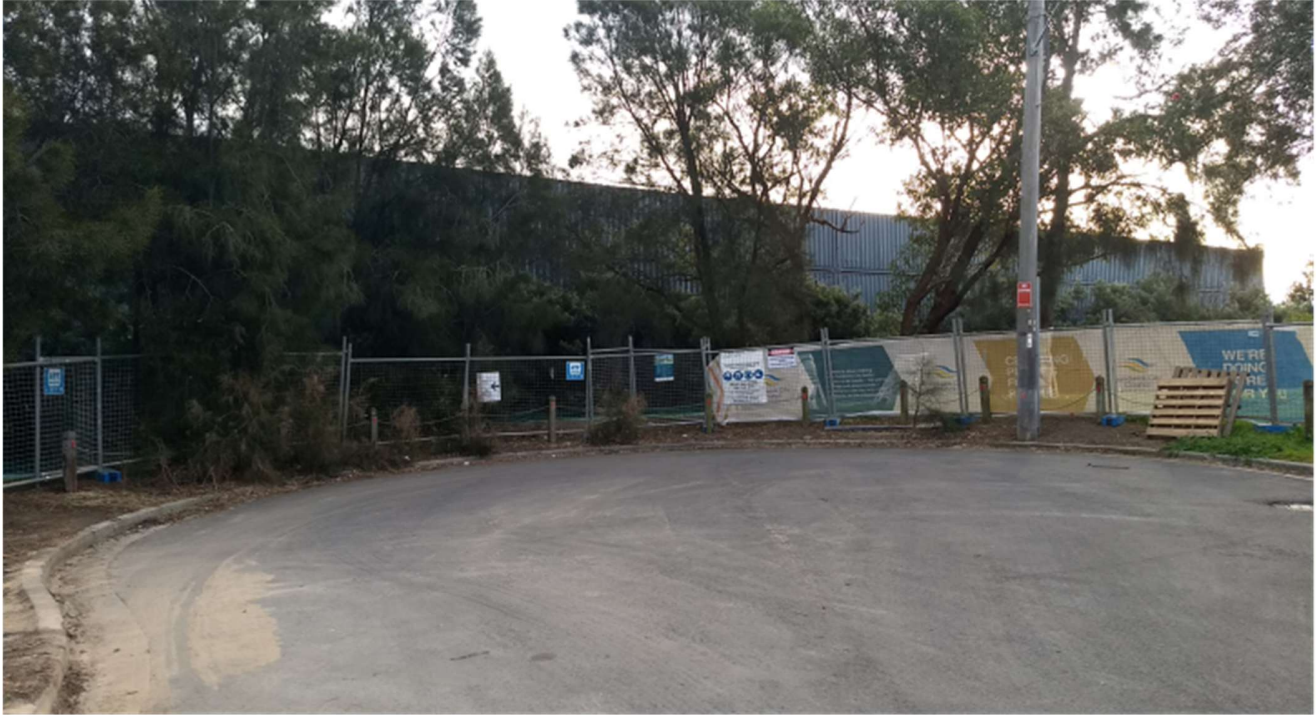
Figure 4 View of northern section of container noise wall following demolition of the B7 reel store - May 2020
