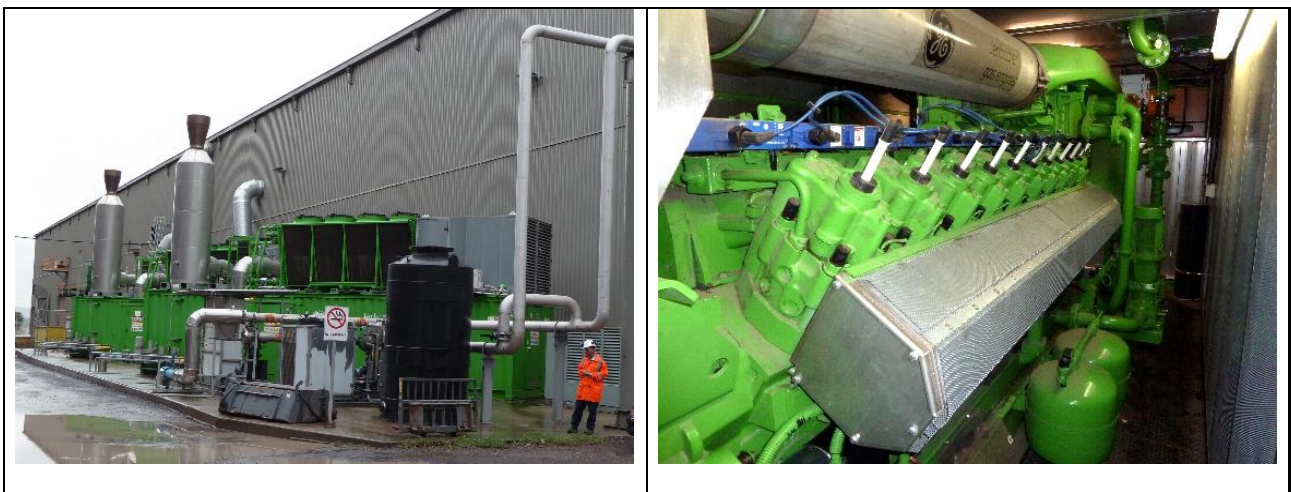
Double Jenbacher 1400 kW CHP
