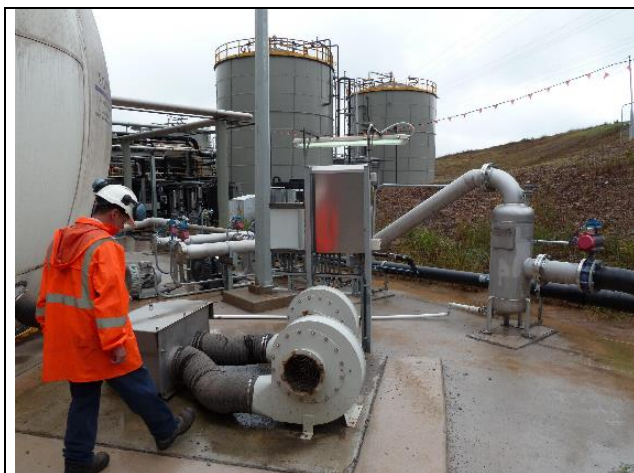
Air blowers of biogas holding tank
