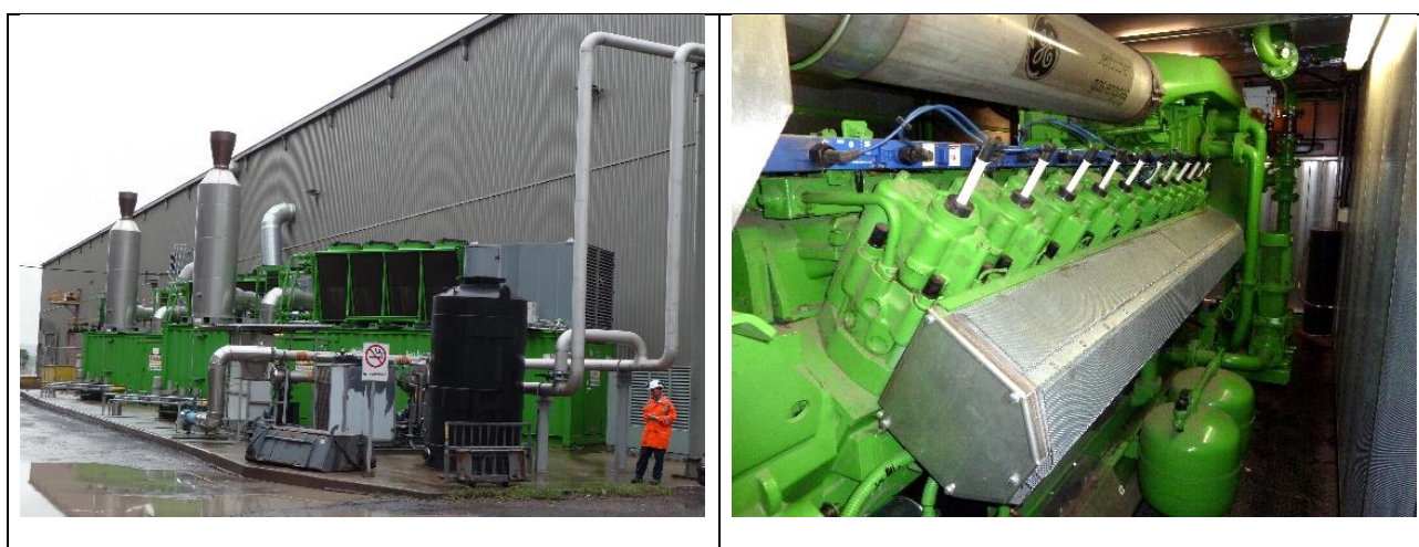
Figure 3. Double Jenbacher 1400 kW CHP
