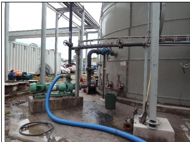
AC2 extraction pump
