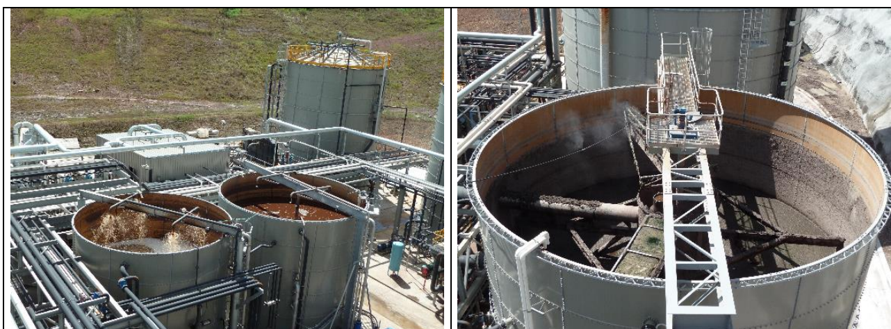
Aerial view of the 2 SBR
