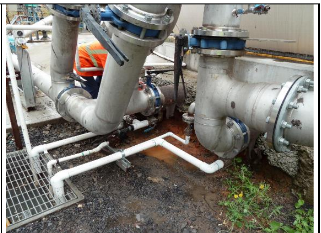
Condensate bleed valves
