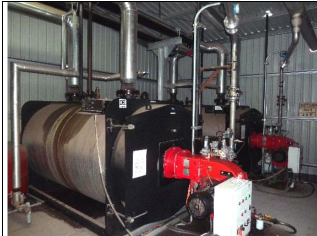
Dual fuel heating system
