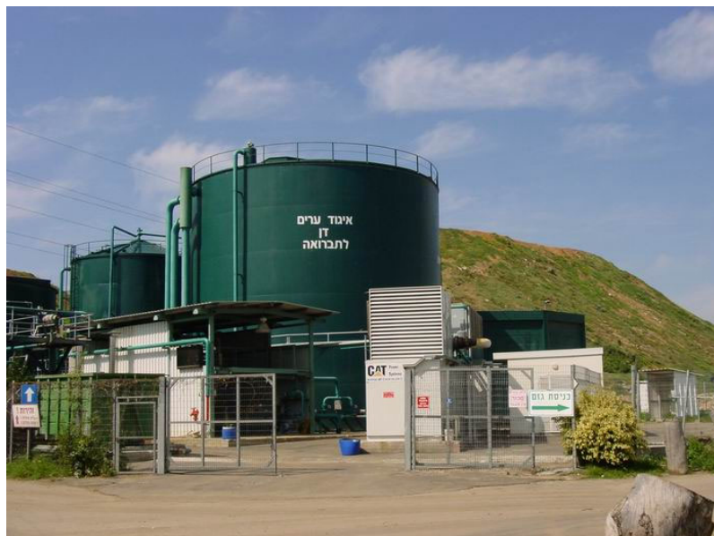
Figure 5-9 Biological treatment plant
