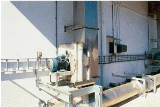
Figure 5-18 Air supply system
