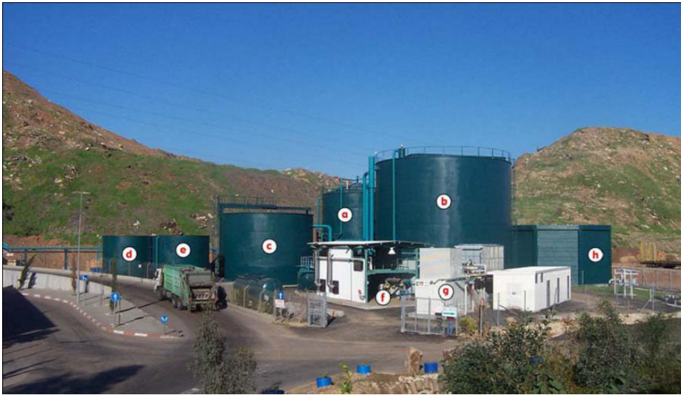
Figure 1-6 Tank farm at Tel Aviv facility (photo)
