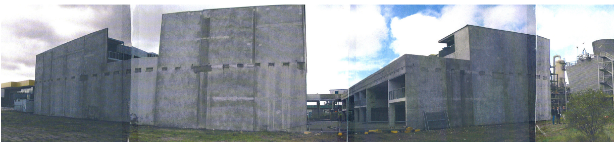
Figure 7: Existing wall along eastern boundary of the site (note people in bottom right corner for scale).
