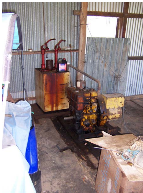
Photograph F: Diesel power generator at Spring Flat, with oil staining on ground.
