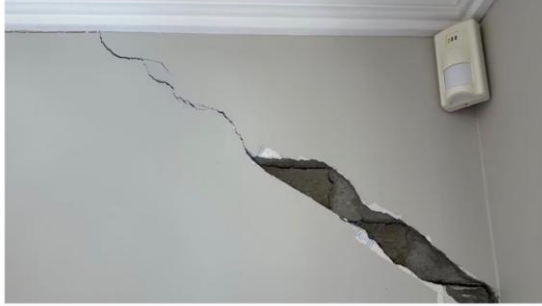
Cracks which developed in a home 200 metres away from a construction site in Rose Bay, which the resident claims are linked to excavation. Picture: Rose Bay Residents Action Group
