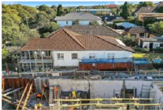
The front rooms of a house next to a development site on Wilberforce Avenue in Rose Bay caved after the excavation of a single storey. Ray White
