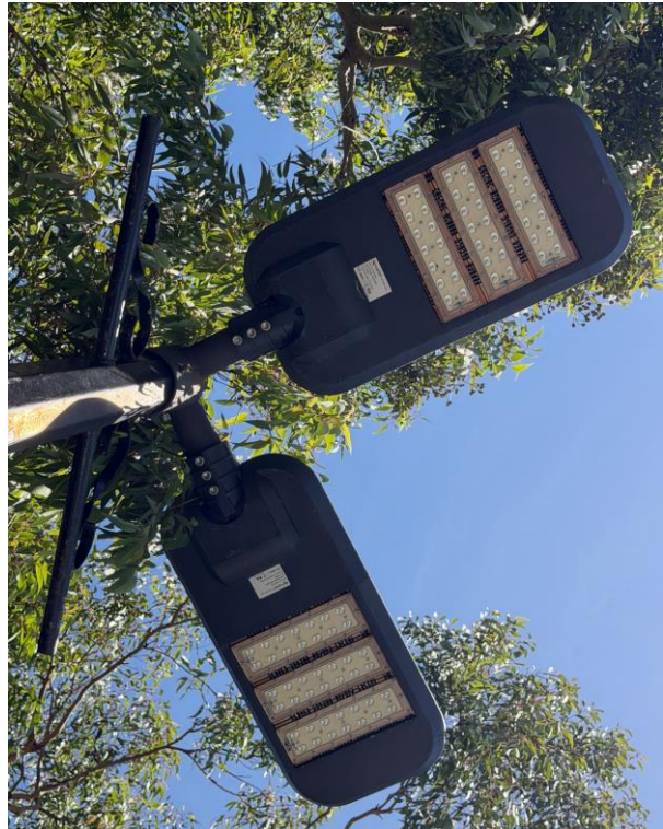
Figure 4 – St Ives Shopping Village Carpark Lighting
