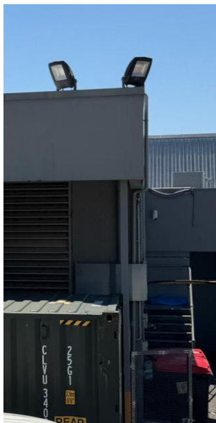
Figure 5 – COLES loading dock Lighting
