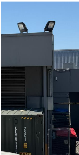
Figure 4 – COLES loading dock Lighting
