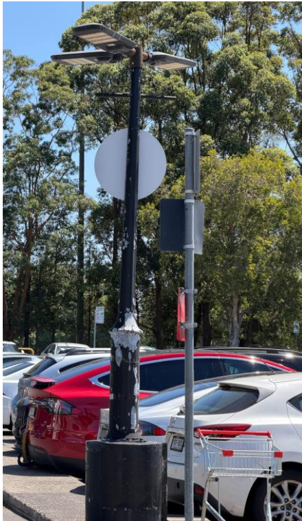
Figure 2 – St Ives Shopping Village Carpark Lighting
