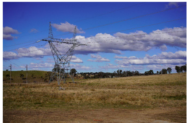
FIGURE 5-2 TRANSMISSION LINES NORTH OF THE SITE
