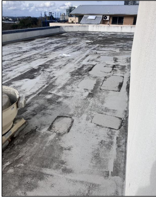
Photograph 61: South Tower, Level 5, open rooftop area, roof surface, exposed waterproofing membrane, SMF detected by analysis.
