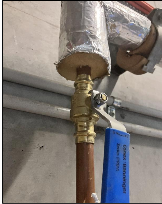
Photograph 57: South Tower, Level 5, Plant Room, accessible water pipe work, bulk insulation, SMF identified visually.
