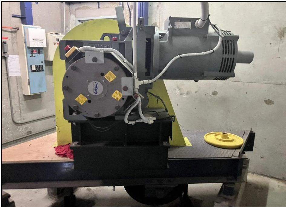
Photograph 48: South Tower, Level 5, Lift Motor Room, lift plant, internal components (e.g. friction pads), inaccessible.
