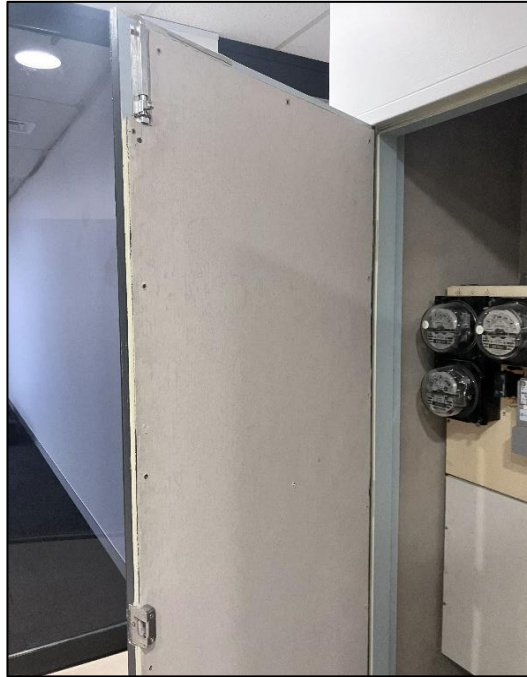
Photograph 35: South Tower, Level 4, lift foyer, EDB cupboard, doors, fibre cement linings, no asbestos detected by analysis.
