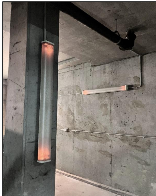
Photograph 66: South Tower, Basement, fluorescent light fittings, internal components, PCB (suspected).
