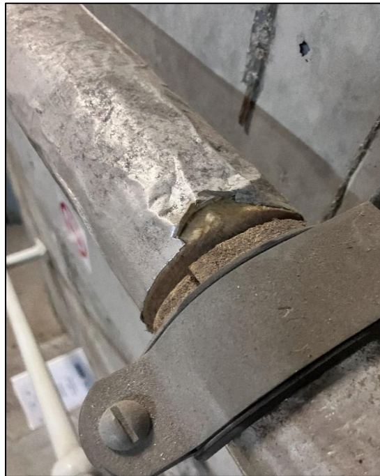
Photograph 58: South Tower, Level 5, Plant Room, accessible water pipe work, bulk insulation, SMF identified visually.
