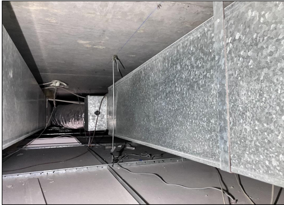
Photograph 31: South Tower, building in general, air conditioning duct work at re-heat elements, duct insulation, inaccessible.
