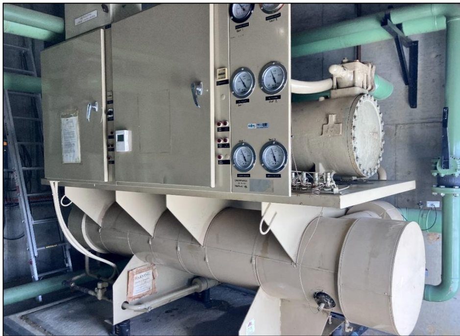
Photograph 46: South Tower, Level 5, Plant Room, boiler unit(s), bulk insulation, inaccessible.
