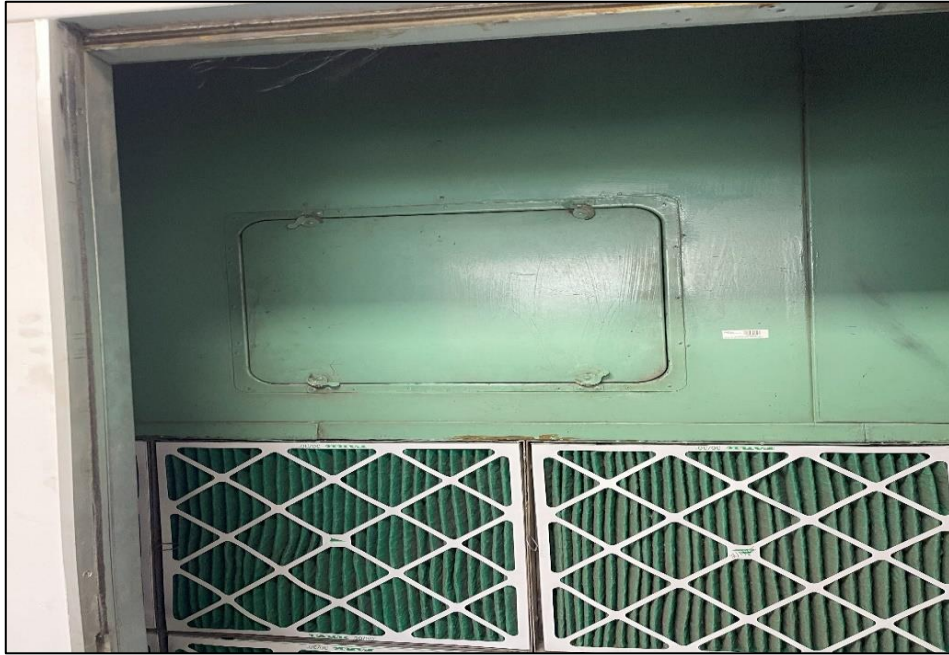
Photograph 11: North and South Tower, building generally, plant room, air handling duct work generally, SMF (suspected).
