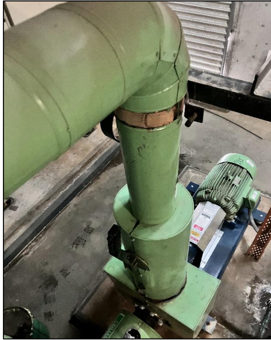
Photograph 59: South Tower, Level 5, Plant Room and open roof area, sheathed pipes and plant, bulk insulation, SMF and foam identified visually.
