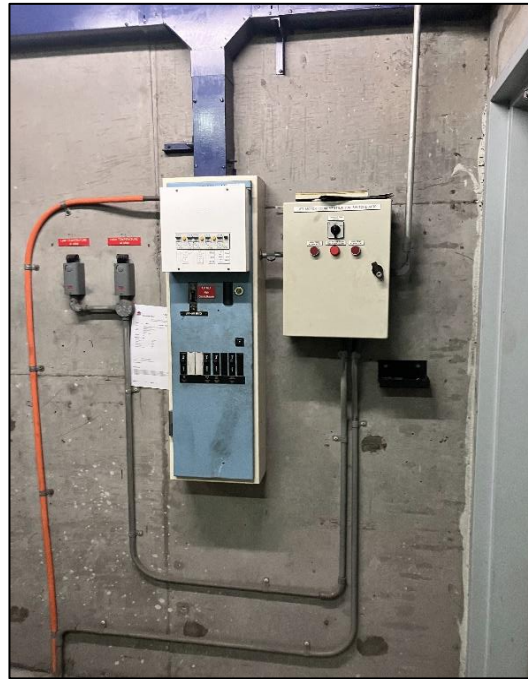
Photograph 49: South Tower, Level 5, Lift Motor Room, electrical panels, internal components (e.g. backing boards), inaccessible.
