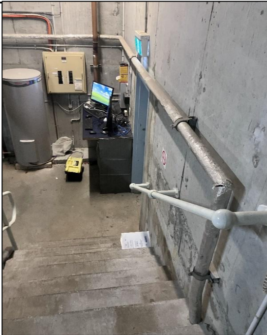
Photograph 56: South Tower, Level 5, Plant Room, accessible water pipe work, bulk insulation, SMF identified visually.
