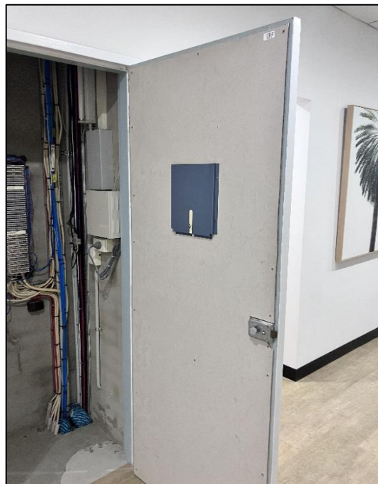
Photograph 34: South Tower, Level 3, lift foyer, Comms cupboard, fibre cement linings, no asbestos detected by analysis.
