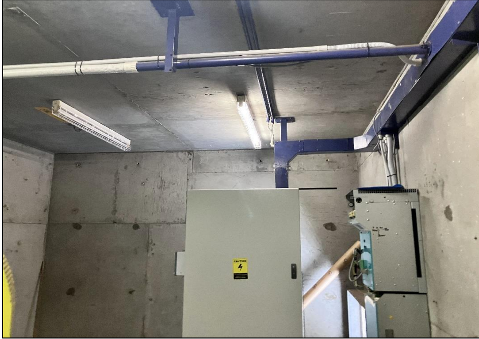
Photograph 63: South Tower, Level 5, Lift Motor Room, fluorescent light fittings, internal components, PCB (suspected).
