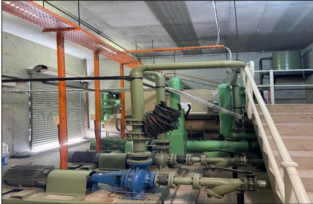
Photograph 5: North and South Tower, Level 5, Plant Room, sheathed pipes and plant, bulk insulation, SMF and foam identified visually.
