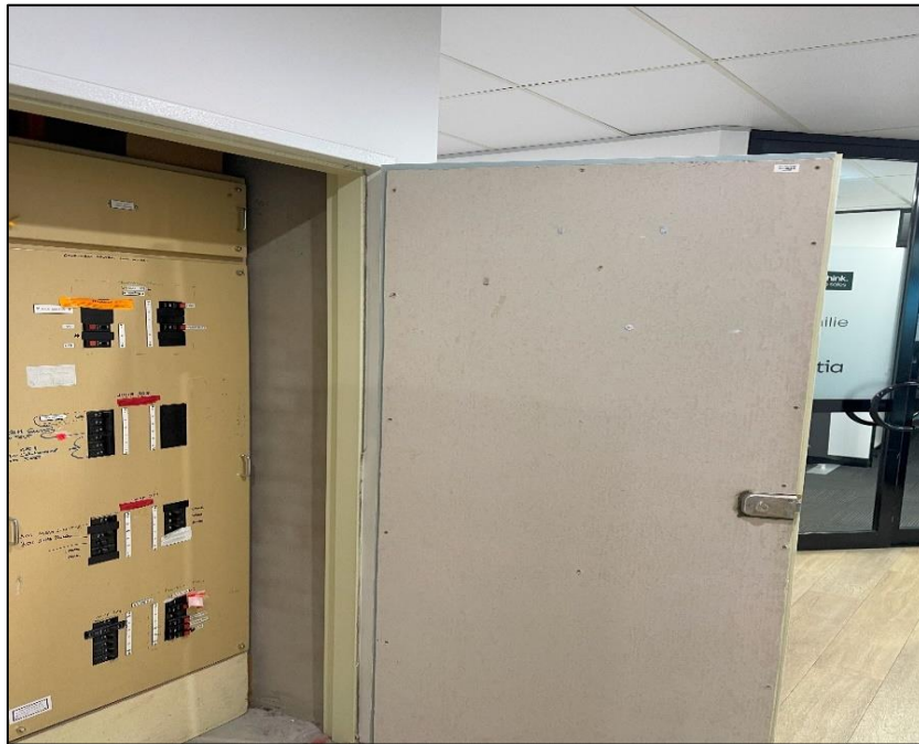
Photograph 12: North Tower, level 3, lobby, EDB cupboard door lining, fibre cement sheeting, no asbestos detected by analysis.
