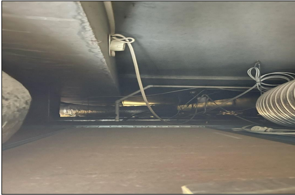
Photograph 19: North Tower, unit 301, ceiling cavity, settled dust / debris, elevated lead concentration detected.
