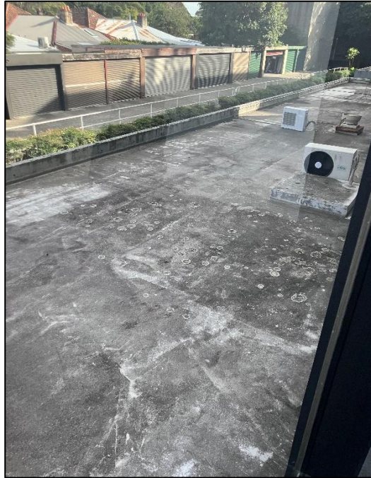
Photograph 33: South Tower, exterior, Ground Level to Level 1, open roof top areas (northeast and southwest), waterproofing membranes, inaccessible.
