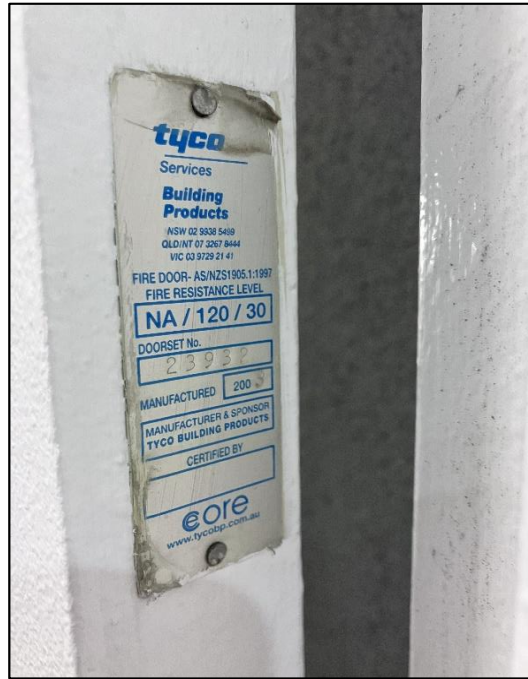
Photograph 39: South Tower, fire stairs and tunnels generally, fire doors c. 2000's (e.g. typically "Tyco" or "DEM" brand) , insulation, suspected non-asbestos.
