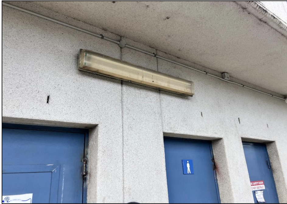
Photograph 65: South Tower, Ground Level, exterior façade, fluorescent light fittings, internal components, PCB (suspected).
