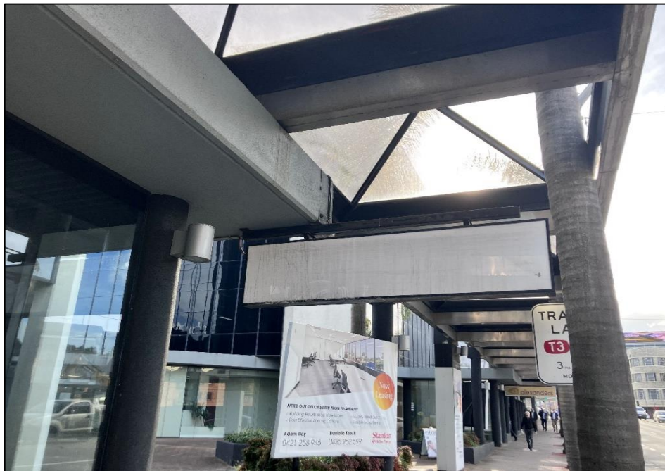
Photograph 64: South Tower, Ground Level, exterior façade, fluorescent light fittings, internal components, PCB (suspected).
