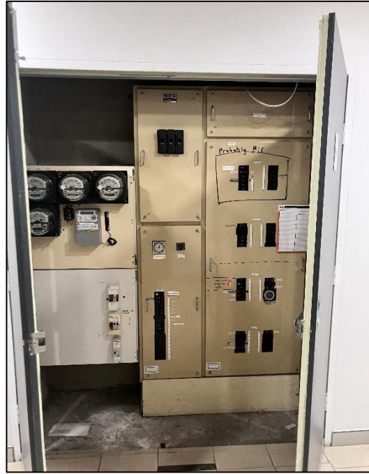
Photograph 37: South Tower, Levels 1 to 4, lift foyer, EDB cupboard, electrical cabinets, internal components, inaccessible.
