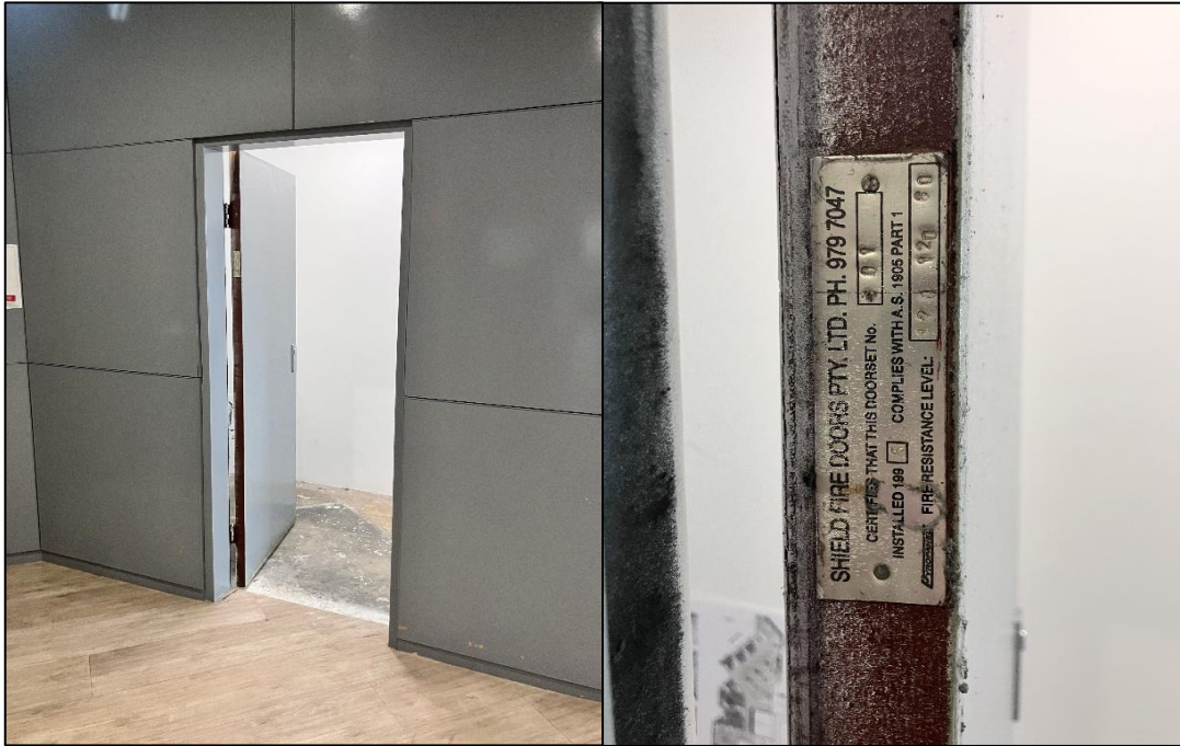
Photograph 51: South Tower, Ground Level, lift foyer, internal entrance to Unit 2, "Shield" fire door (c. 1995), insulation, suspected asbestos.
