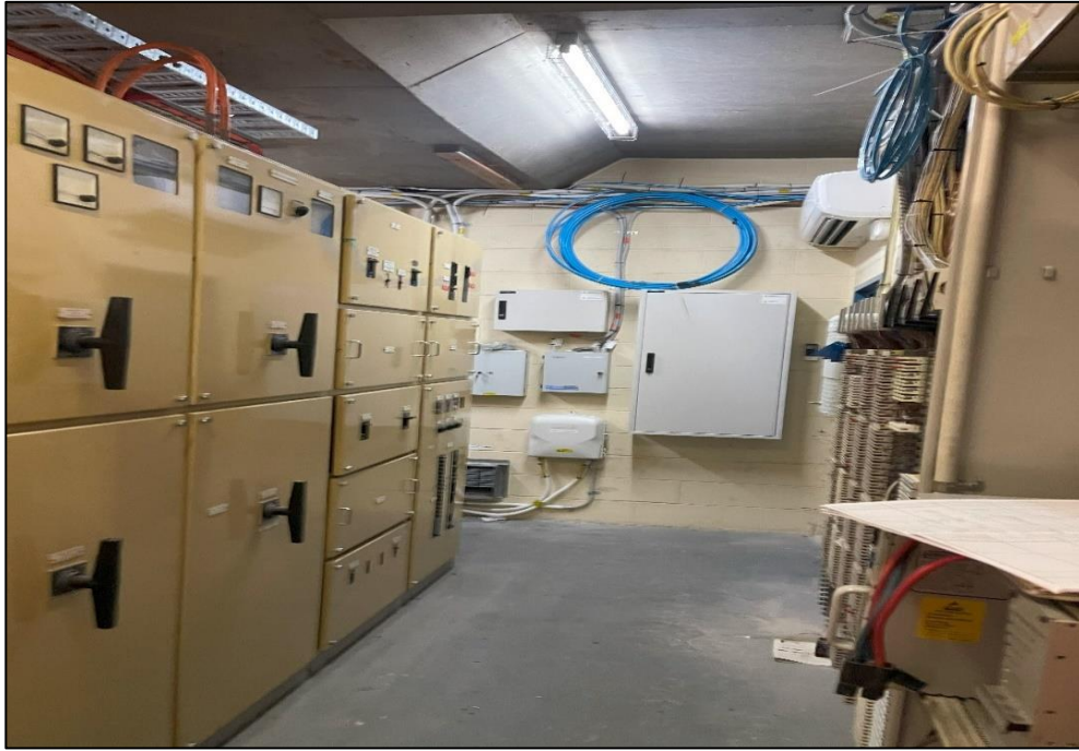
Photograph 29: Basement car park, services room, materials in general, limited access, suspected non-asbestos.
