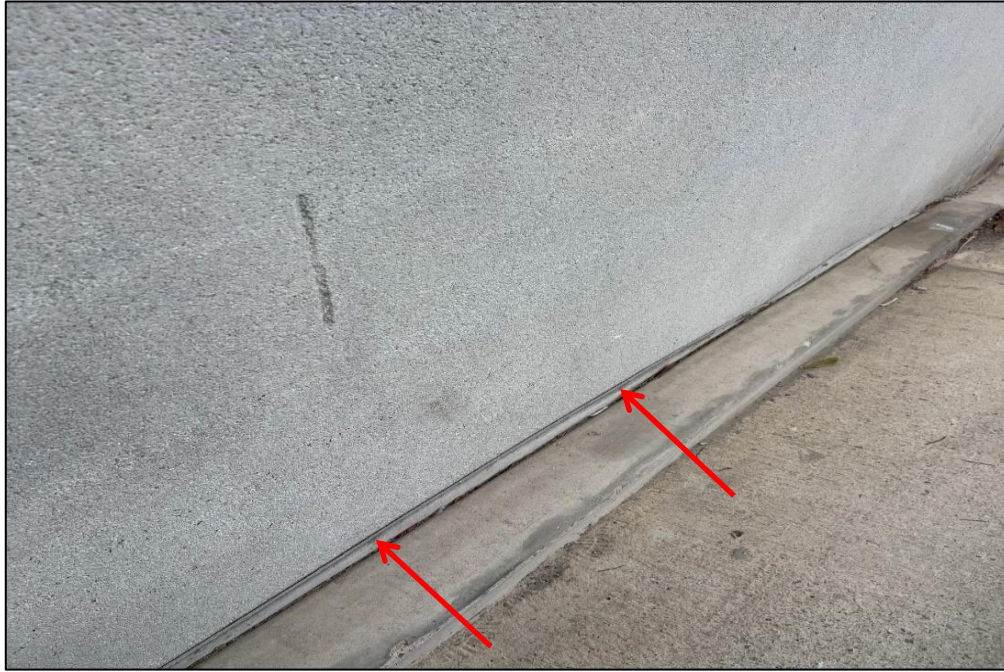
Photograph 3: North Tower, exterior, western end, base of wall, expansion gap, fibrous board, no asbestos detected by analysis.
