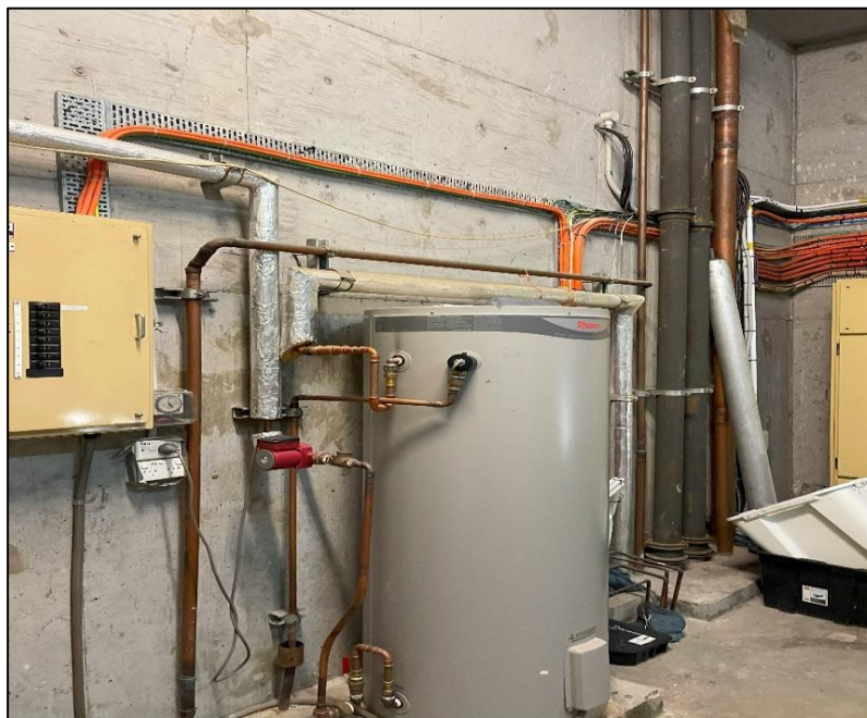
Photograph 20: North Tower, rooftop, plant room, water heater, insulation materials, SMF (suspected).
