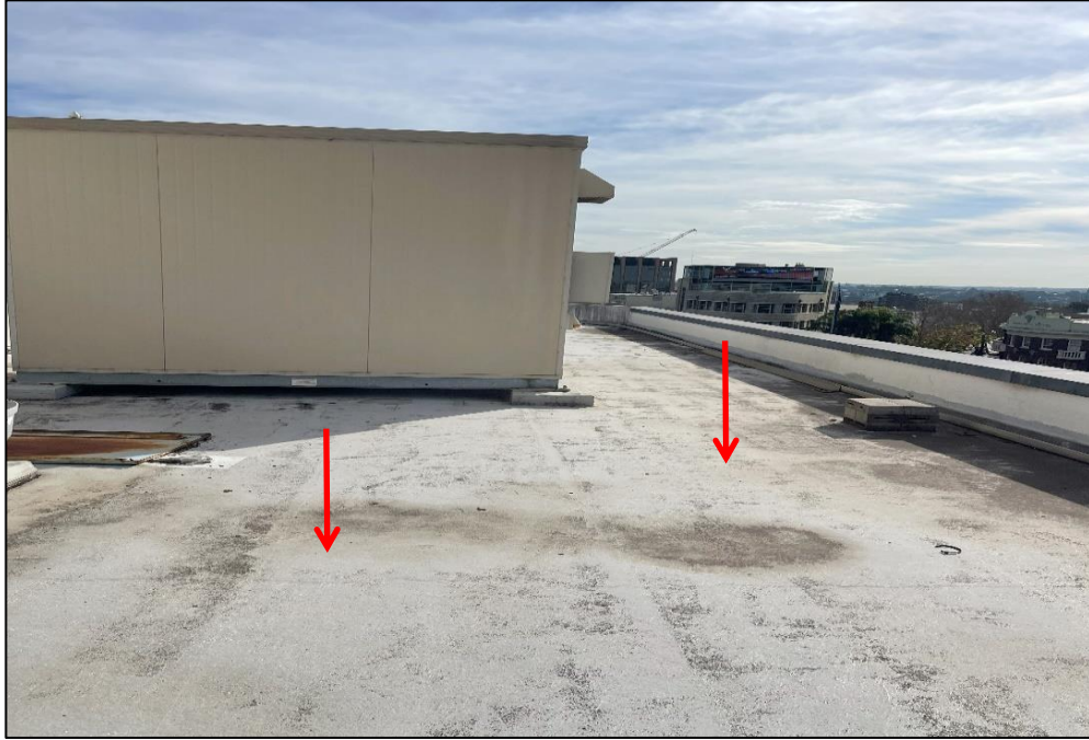
Photograph 7: North Tower, rooftop, exposed waterproof lining, fibrous membrane, no asbestos detected by analysis (SMF detected).
