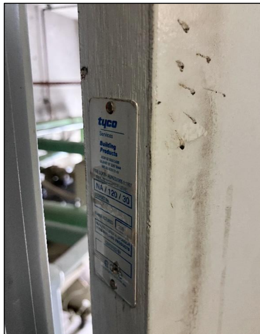
Photograph 50: South Tower, Level 5, Lift Motor Room, "Tyco" fire door (circa 2000's), insulation, suspected non-asbestos.
