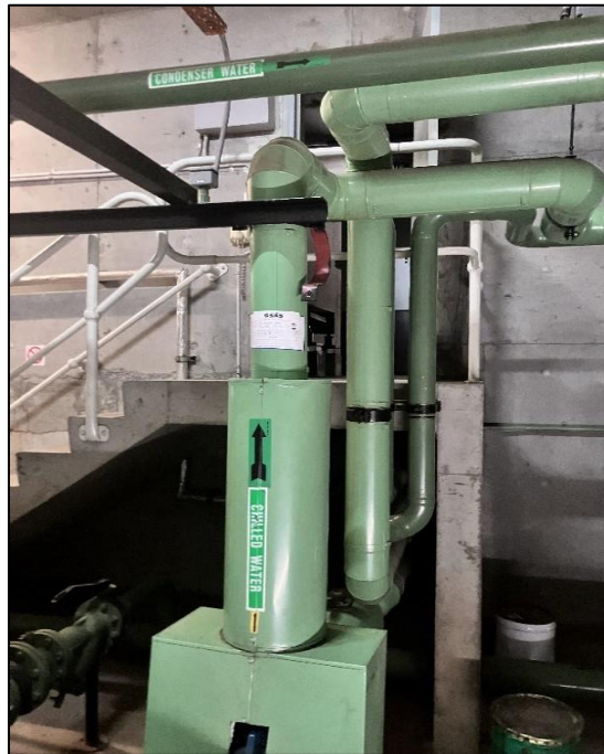
Photograph 60: South Tower, Level 5, Plant Room and open roof area, sheathed pipes and plant, bulk insulation, SMF and foam identified visually.
