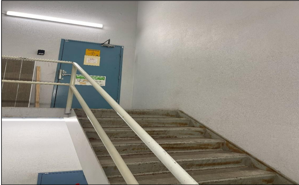
Photograph 17: North Tower, rooftop, fire stairs, white paint to hand rail, blue paint to door and grey paint to wall, negative spot tests.
