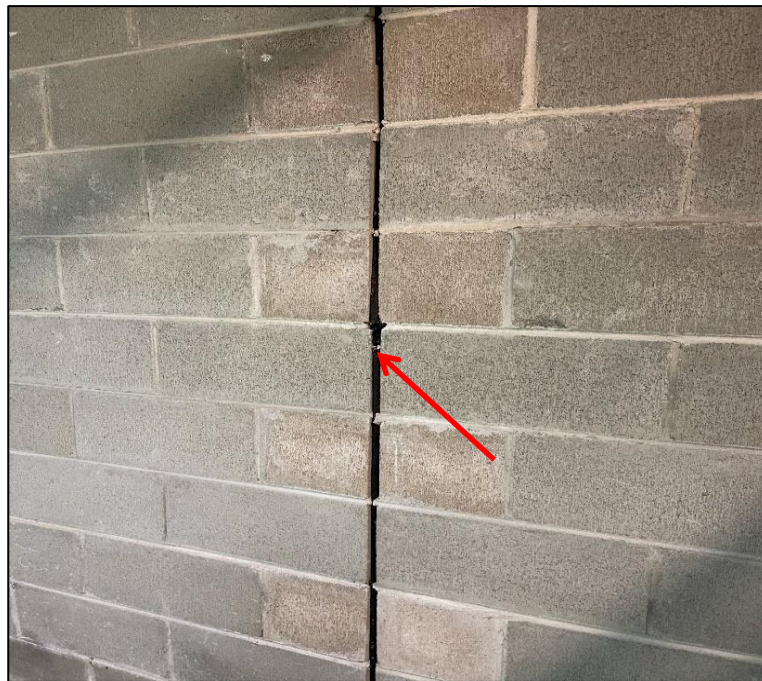
Photograph 28: Basement car park, southern end, wall, expansion gap, lining, no asbestos detected by analysis.
