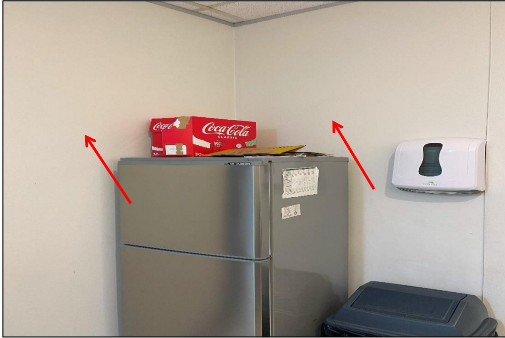
Photograph 9: North Tower, level 4, kitchen, wall lining, fibre cement, no asbestos detected by analysis (SMF detected).
