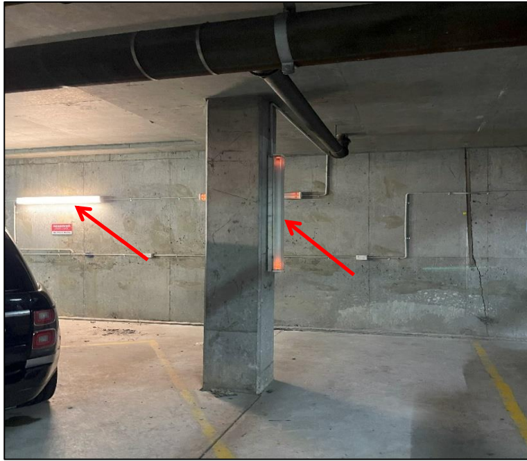
Photograph 23: Basement car park, fluorescent light fittings, internal components, PCB (suspected).
