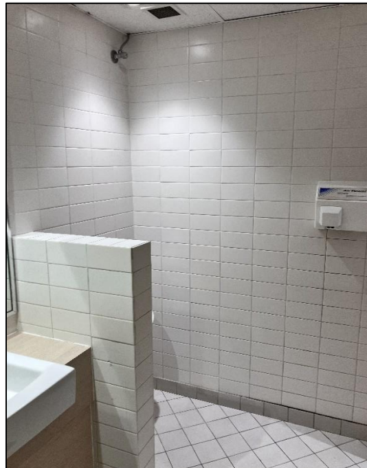
Photograph 40: South Tower, Levels in general, lift foyers, amenities generally, below ceramic floor and wall tiles, substrate, inaccessible.
