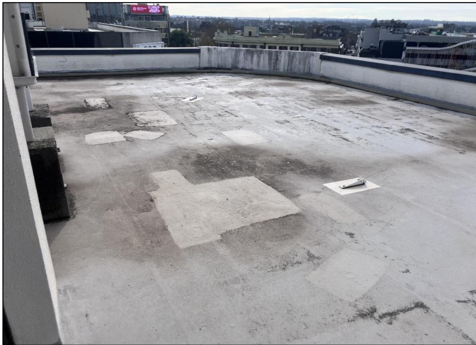
Photograph 42: South Tower, Level 5, open rooftop area, throughout, materials in general, limited access.
