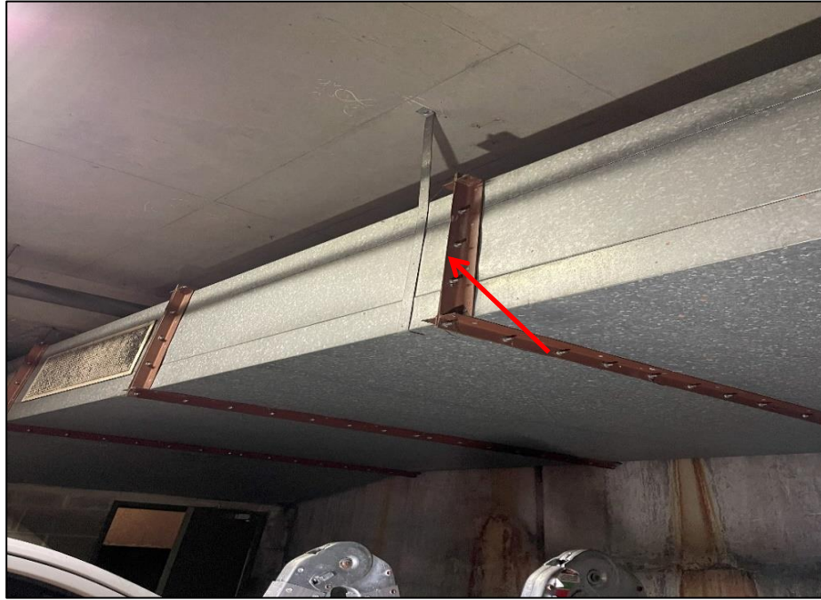
Photograph 27: Basement car park, southern end, air handling duct work, duct joint, mastic, no asbestos detected by analysis.
