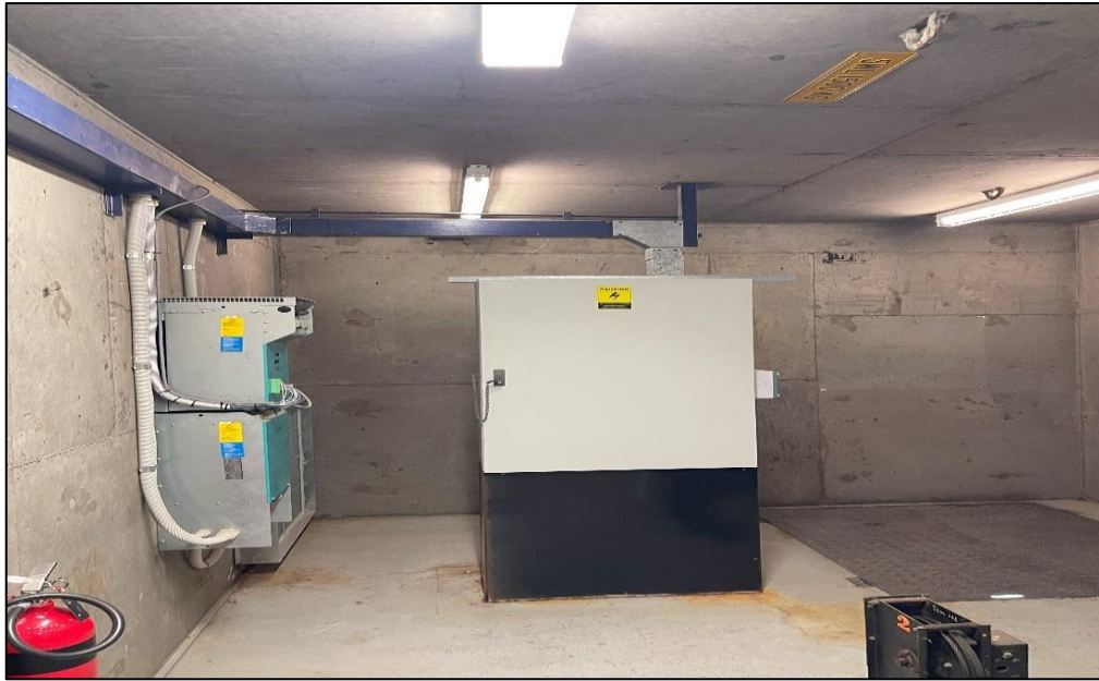
Photograph 21: North Tower, rooftop plant room, fluorescent light fittings, internal components, PCB (suspected).
