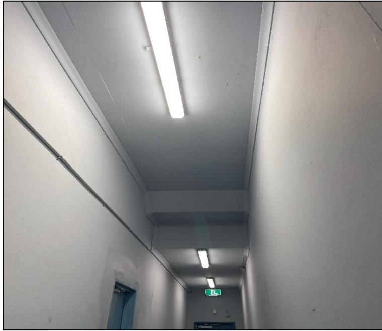
Photograph 25: North Tower, ground level, fire exit corridor, fluorescent light fittings, internal components, PCB (suspected).
