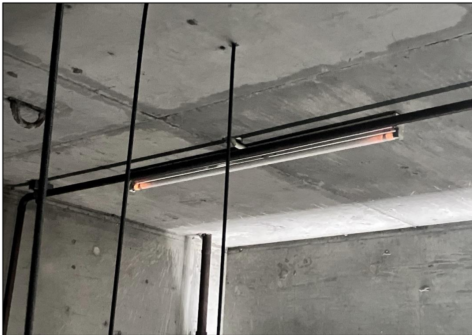
Photograph 62: South Tower, Level 5, Plant Room, fluorescent light fittings, internal components, PCB (suspected).
