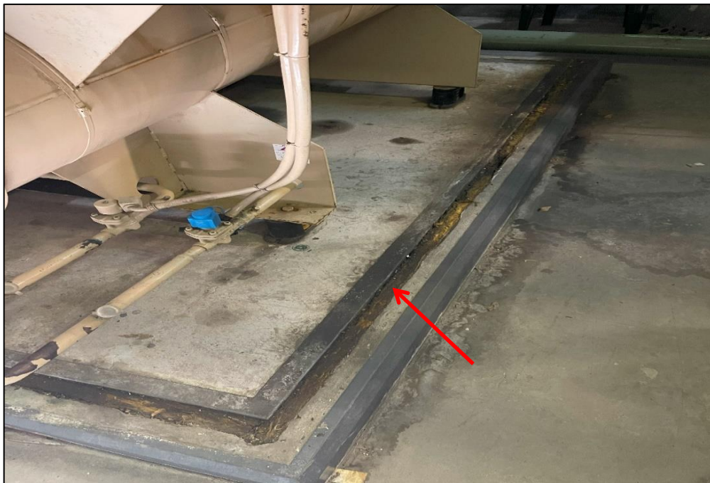
Photograph 6: North Tower, rooftop plant room, floor surface, sealant / mastic, no asbestos detected by analysis.
