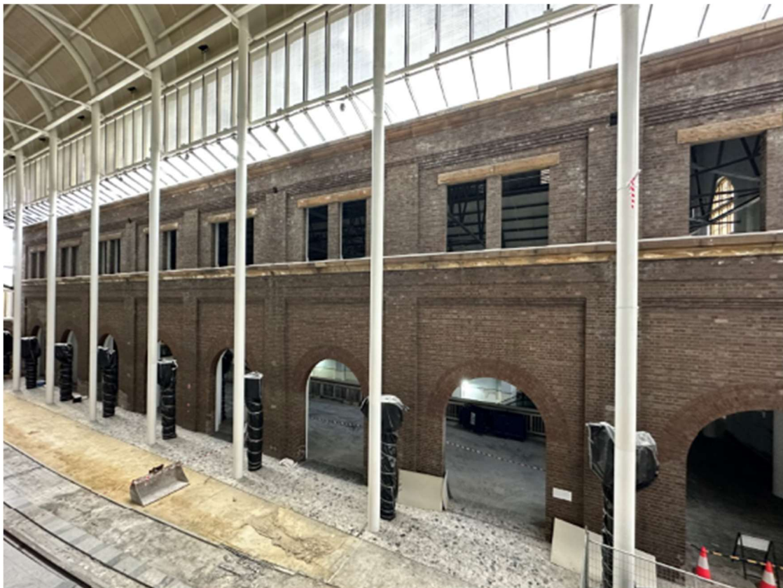
Figure 3: The rhythm and distinctive slenderness of the Galleria portal frames allowed the eastern elevation of the Switch House to retain its presence in such close proximity to the (then) new building. The addition of further structural elements, including potentially a secondary structural system, will diminish the opportunity to recapture this intentional design. (Source: NBRS)
